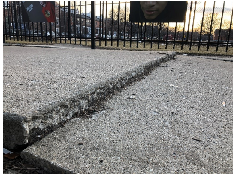
Sidewalk Requiring Repair
