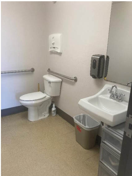
There is only one toilet for staff and public
