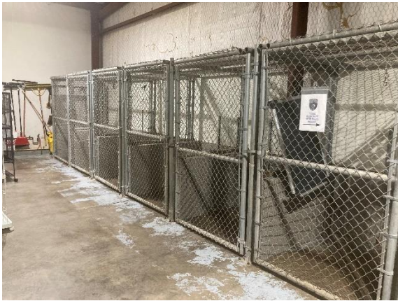
Kennels in the Sally Port are not air conditioned and are in poor condition.
