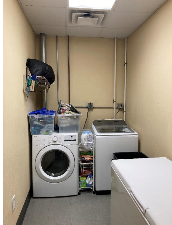
The laundry uses residential laundry equipment, but commercial equipment is preferred.
