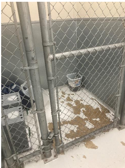
The flooring is peeling up and chain-link fencing is difficult to disinfect.
