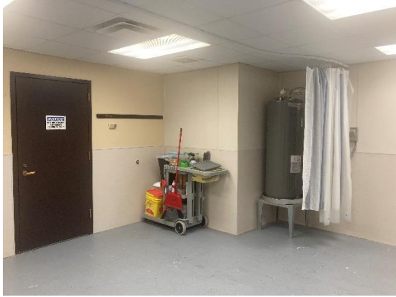
The Cat Room has a water heater exposed in the room. This room also serves as a corridor that dogs are brought through.
