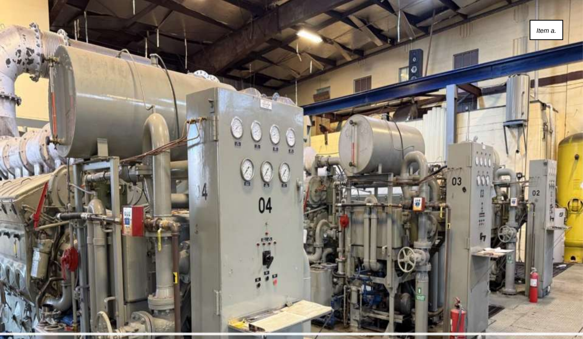
Units 2-4 2 MW Each
