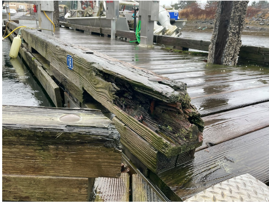
Photo 17. Typical rotten bullrail end
