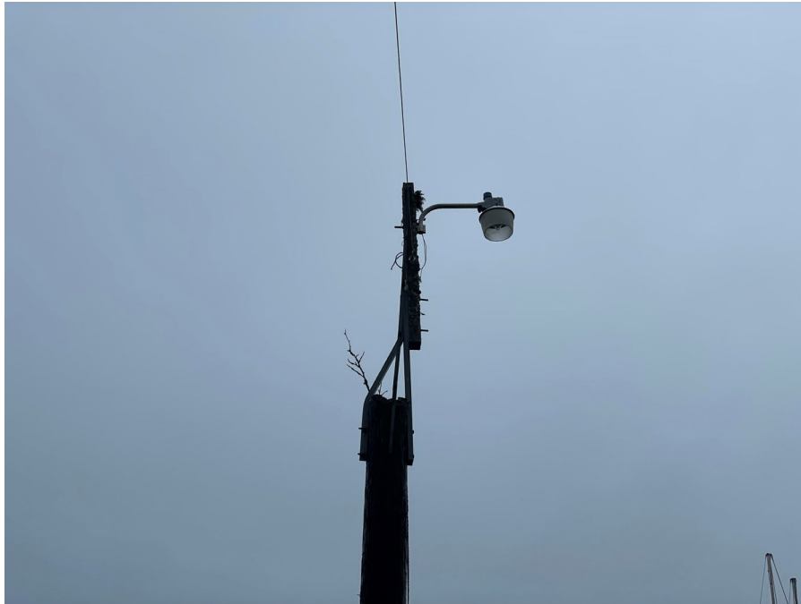
Photo 23. Overhead lighting/small tree growing on pile top
