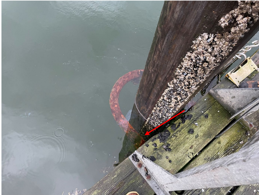
Photo 13. Submerged/corroded pile hoop, mainwalk A
