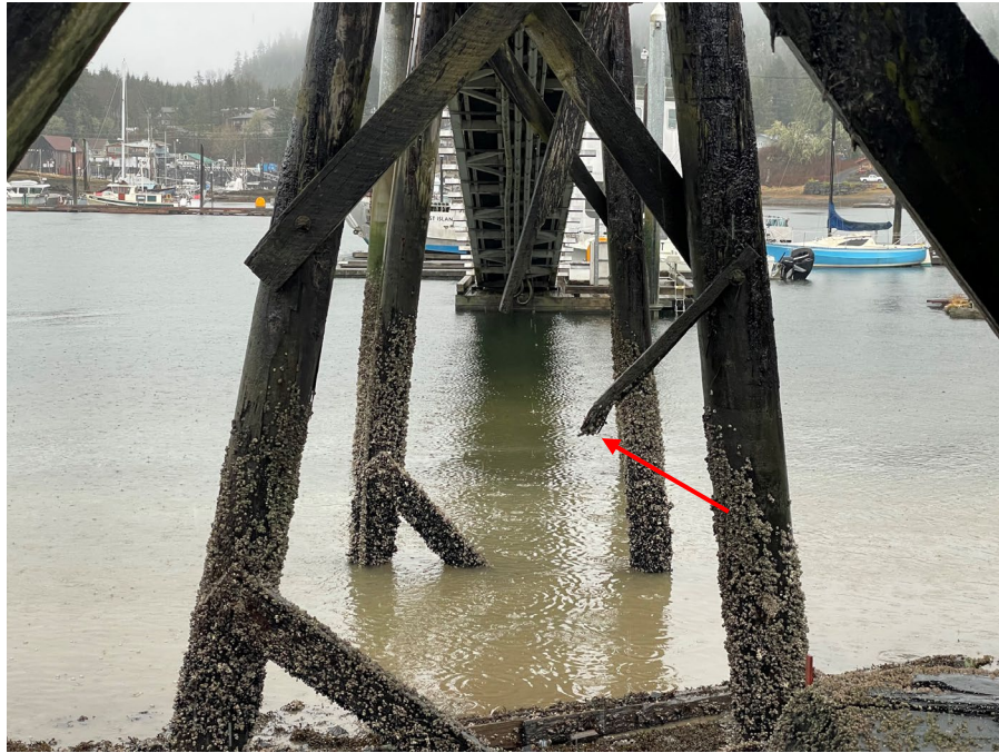
Photo 5. Damaged approach dock cross bracing
