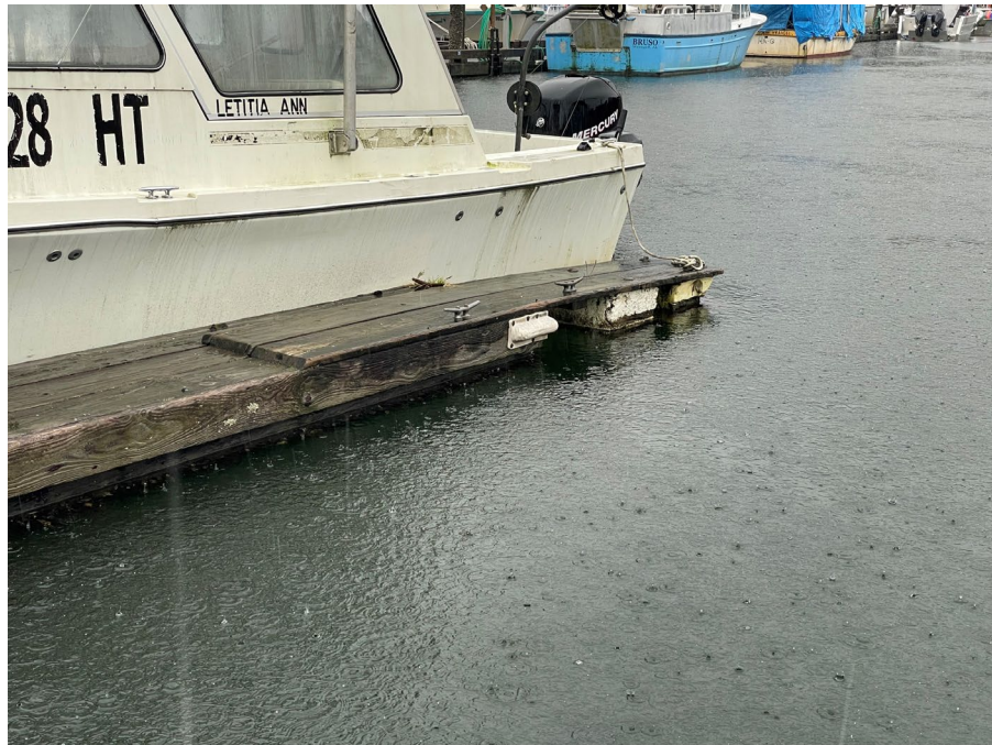
Photo 9. Damaged 2'x17' finger float
