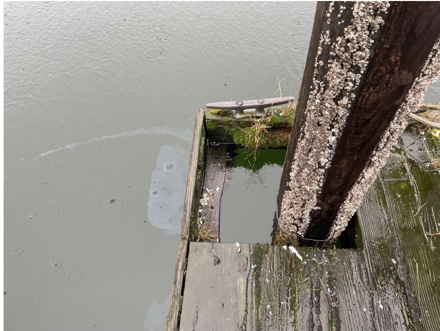
Photo 19. Submerged float timbers/leeching creosote/organic growth/worn pile
