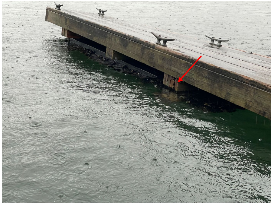
Photo 10. Listing 2'x17' finger float/rotten stringer
