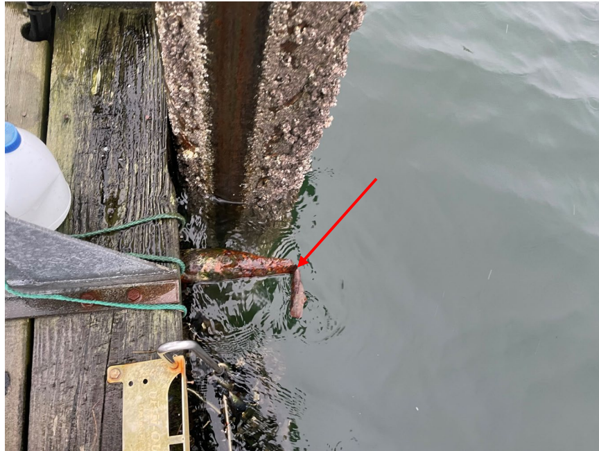
Photo 19. Corroded/missing pile hoop mainwalk E
