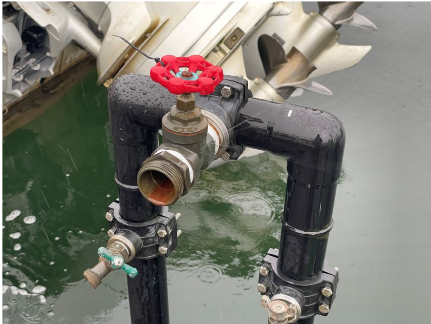
Photo 24. Typical mainwalk water pedestal
