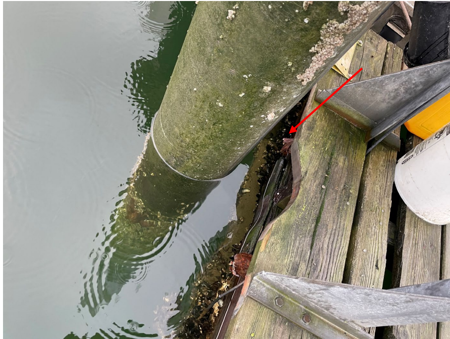
Photo 11. Corroded/missing pile hoop mainwalk A
