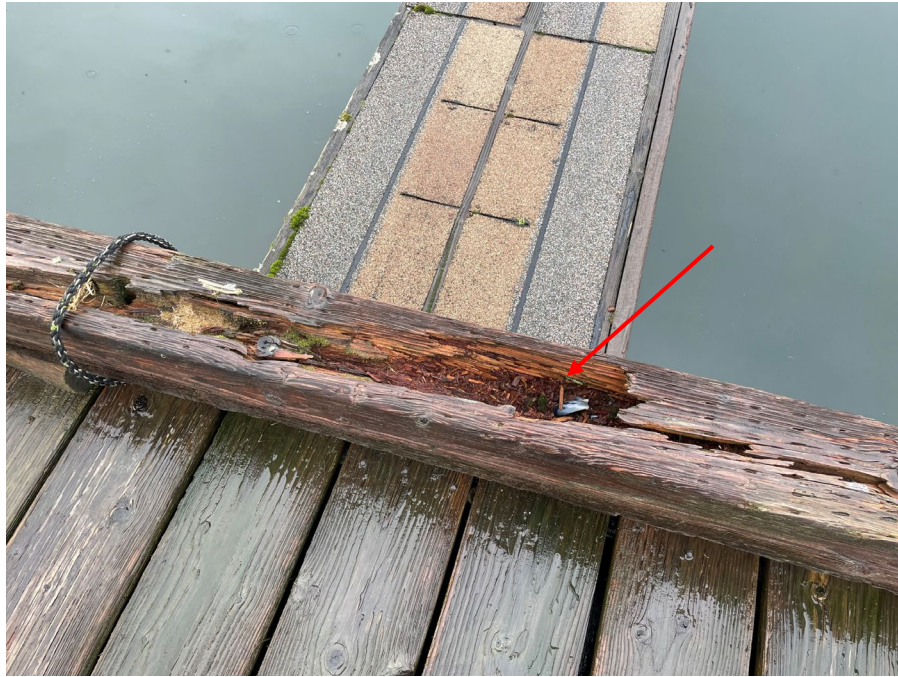
Photo 11. Rotten bullrail on mainwalk A
