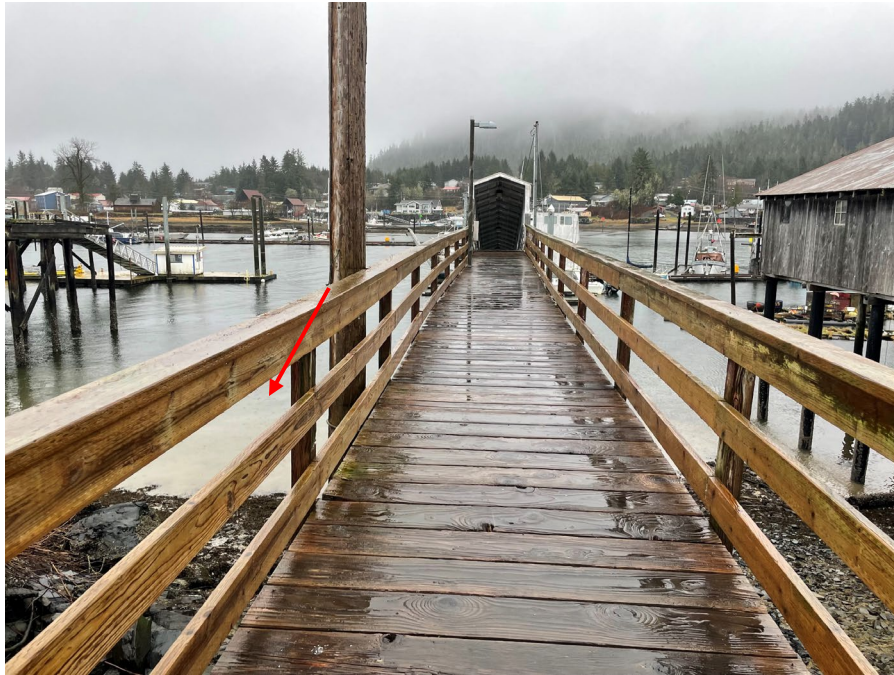
Photo 3. Topside of approach dock/large gap between handrails
