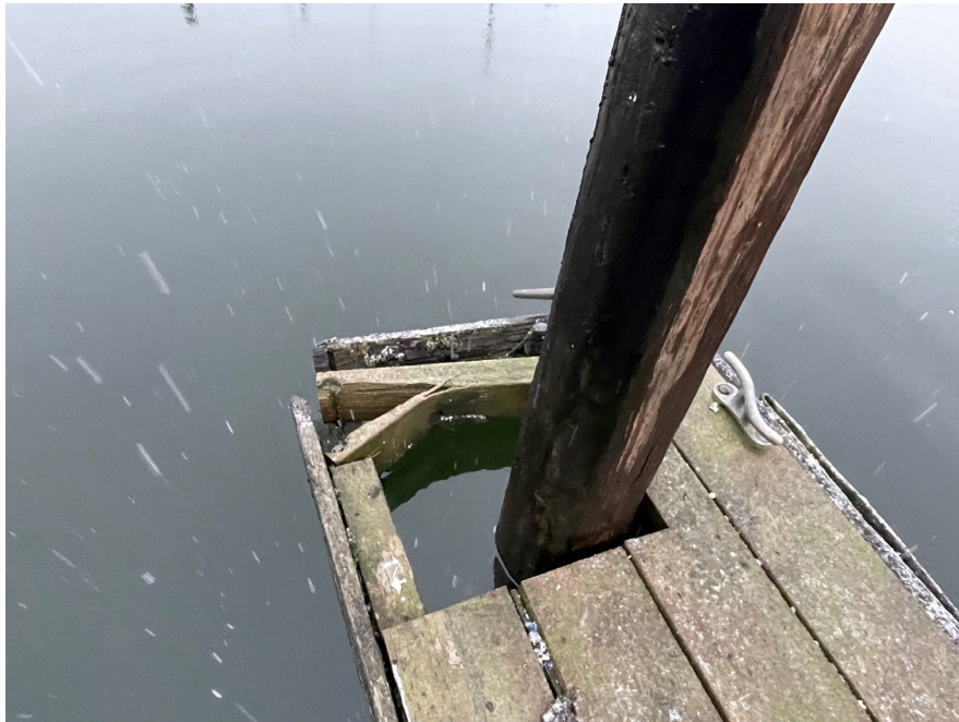
Photo 22. Damaged finger float end
