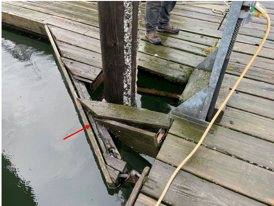
Photo 16. Damaged float timbers/pile hoop mainwalk D
