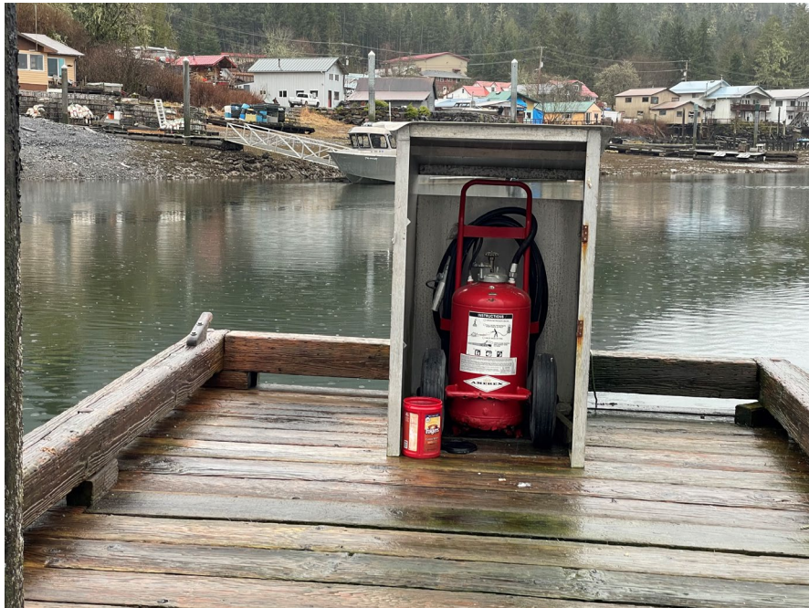
Photo 24. Typical fire extinguisher in cabinet
