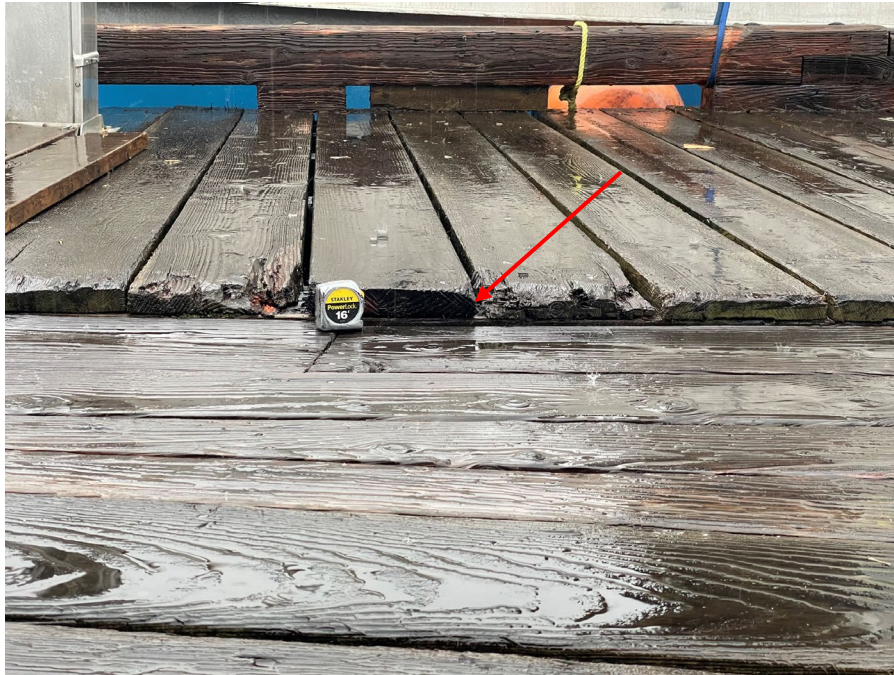
Photo 11. Trip hazard at float to float connection/damaged connection
