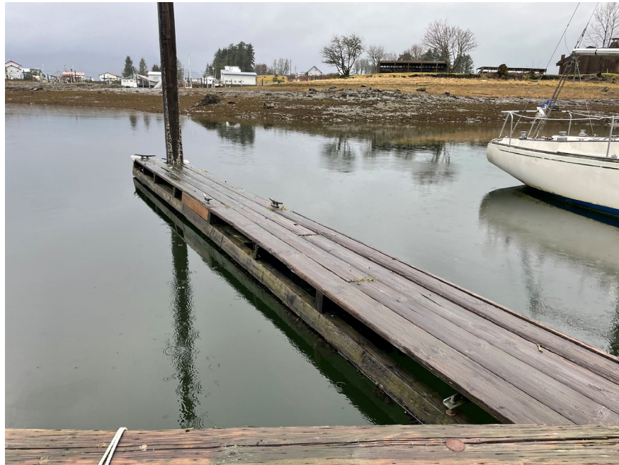
Photo 18. Missing float rubboard/listing issues
