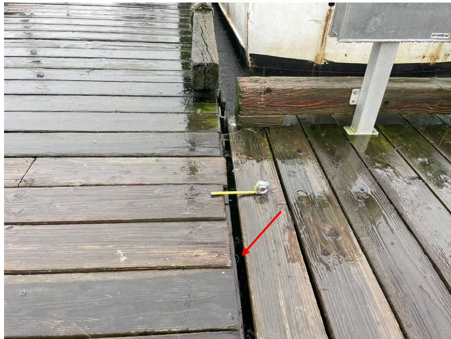
Photo 10. Trip hazard at float to float connection
