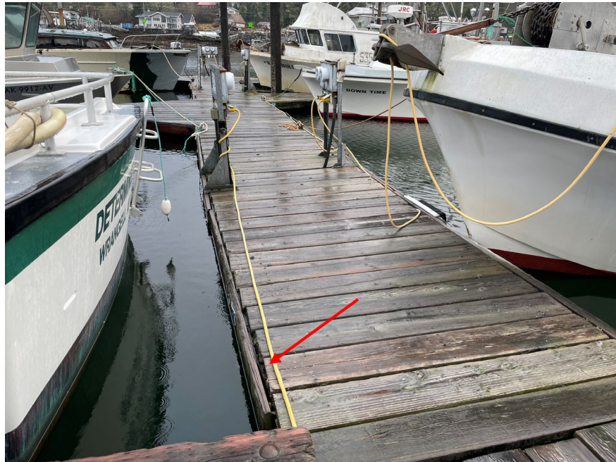
Photo 12. Mainwalk E, low (5") freeboard, float listing
