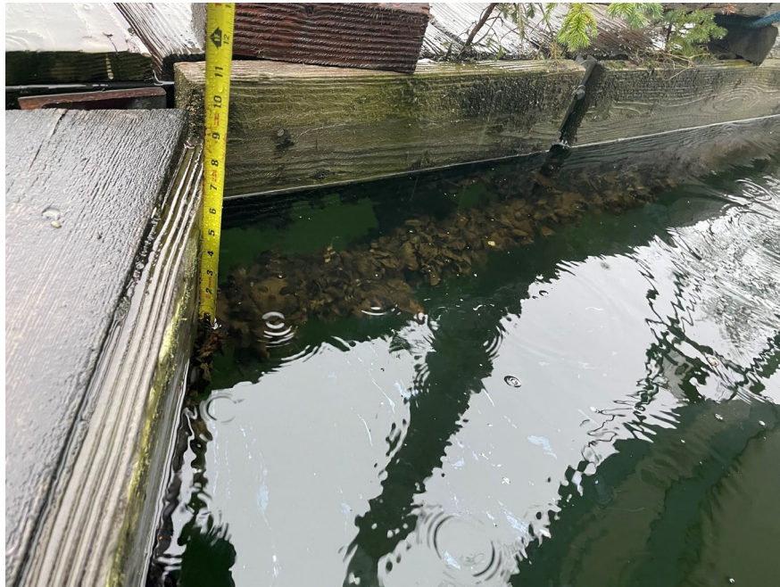
Photo 20. Excessively low float freeboard (5")
