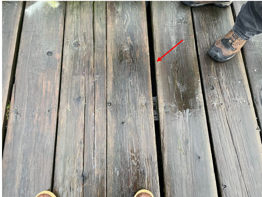
Photo 6. Typical large gap between deckboards
