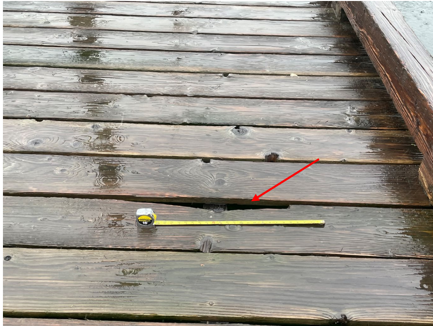
Photo 13. Damaged deckboard/trip hazard
