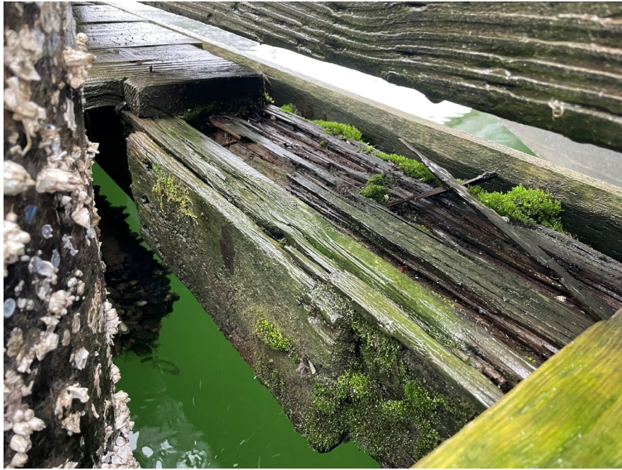
Photo 21. Rotten float stringers
