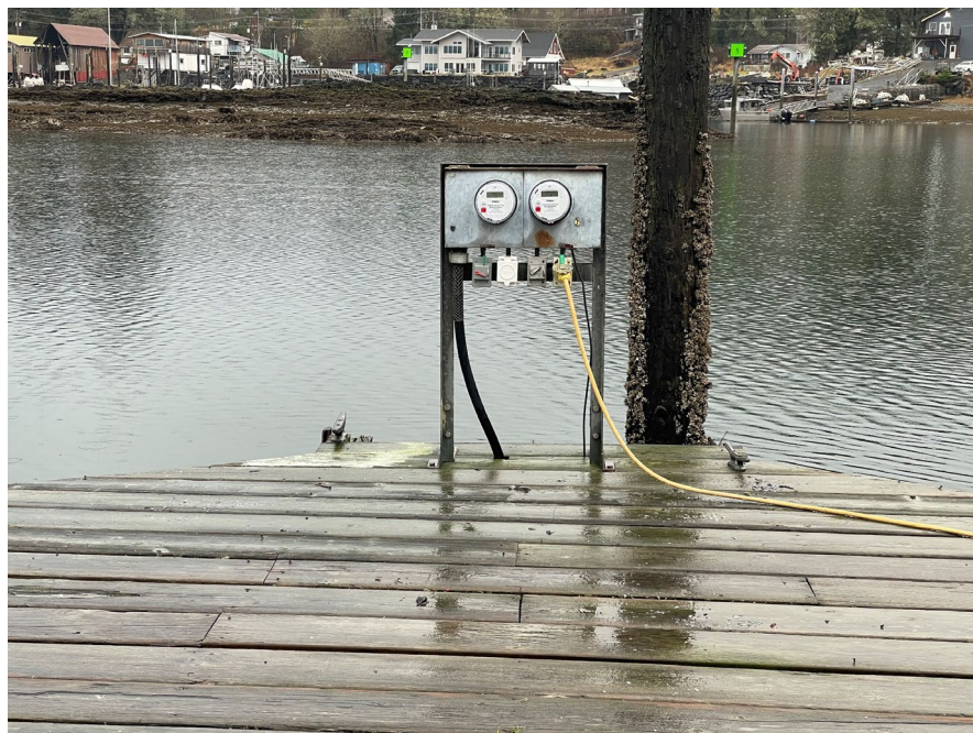
Photo 24. Typical mainwalk electrical pedestal
