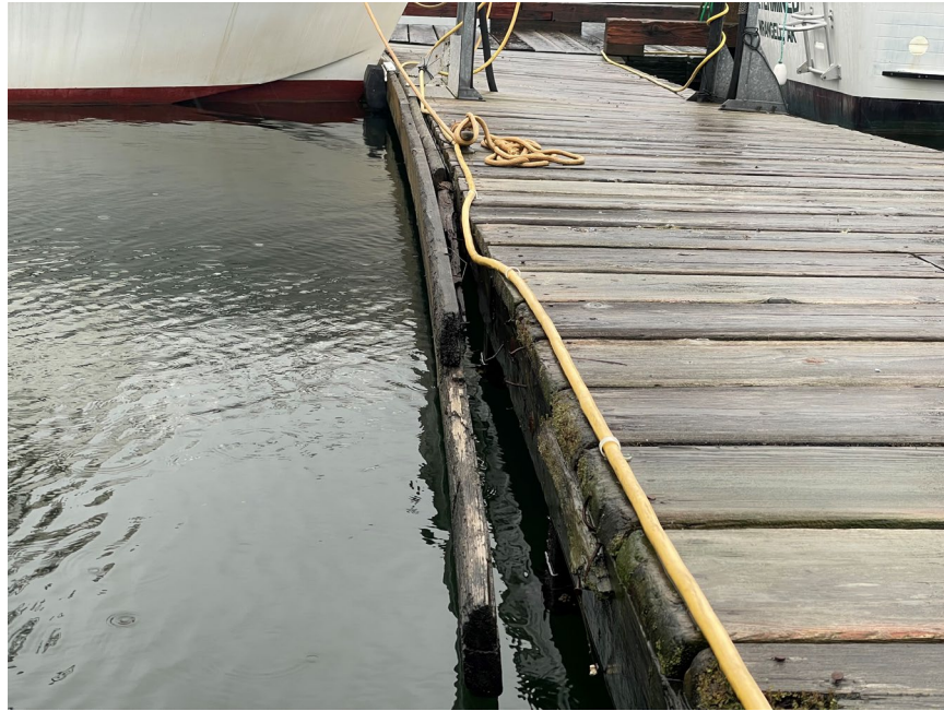
Photo 17. Loose/damaged rubboard/low freeboard
