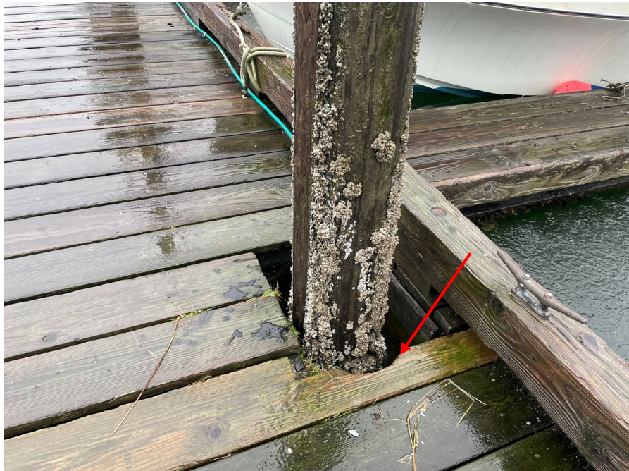
Photo 8. Worn pile/float rubbing
