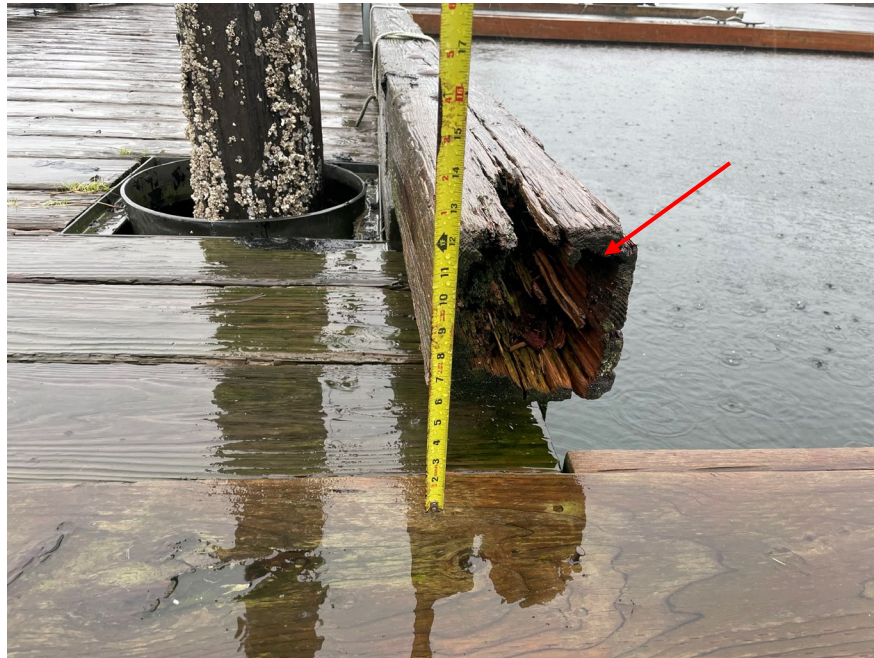
Photo 12. Typical rotten bullrail end on mainwalk A
