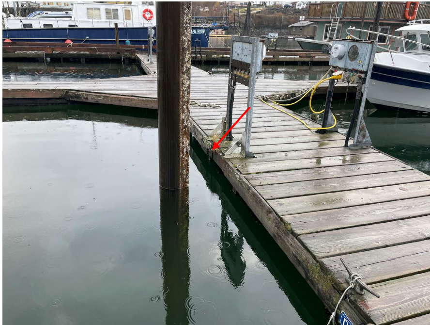
Photo 10. Mainwalk B, missing pile hoop
