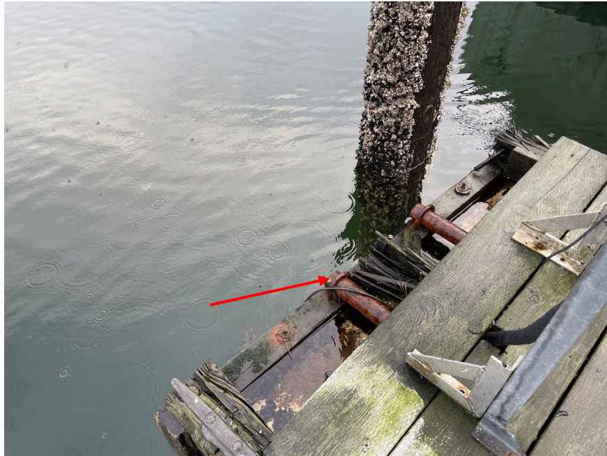
Photo 15. Corroded/missing pile hoop mainwalk C
