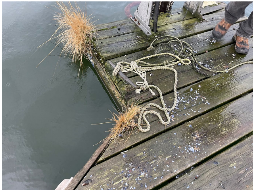
Photo 14. Typical moss/organics/plant growth on float timbers
