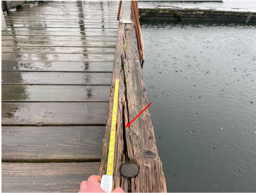
Photo 9. Typical split/rotten headwalk bullrail
