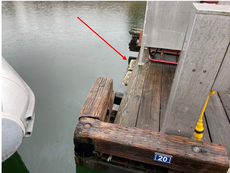
Photo 20. Damaged timbers at end of headwalk float
