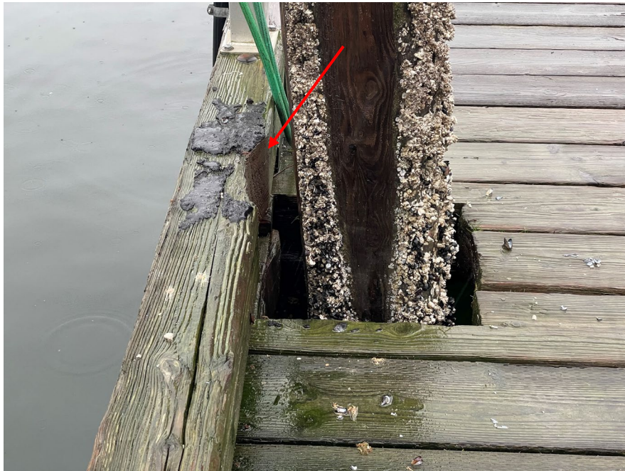
Photo 22. Pile rubbing on float/bullrail
