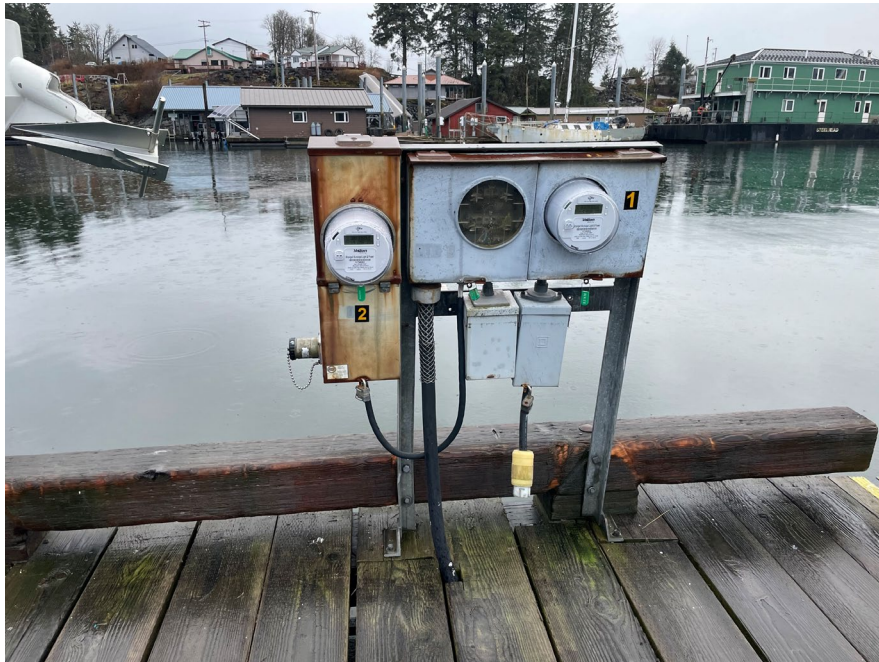
Photo 22. Typical headwalk shore power pedestal
