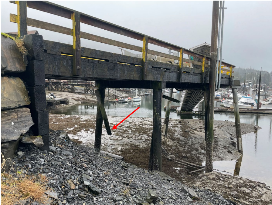
Photo 5. Profile of approach dock/broken cross bracing
