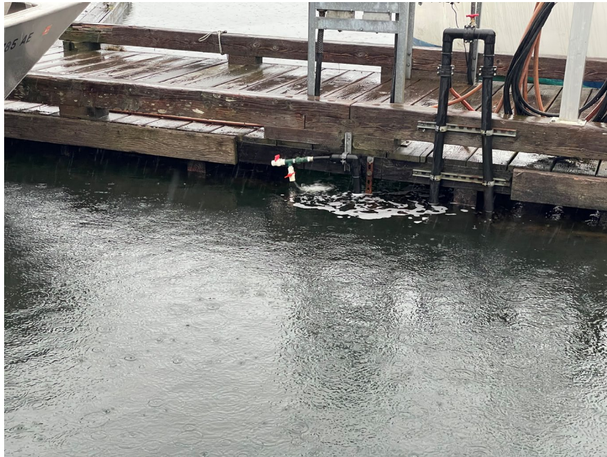
Photo 26. Running water at end of water mainline
