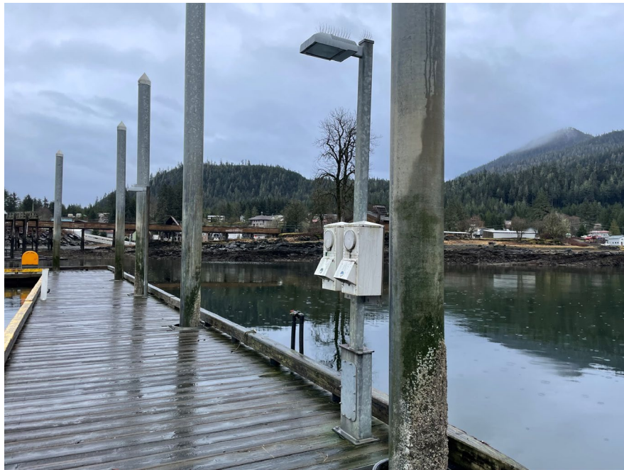
Photo 2. Overview of breakwater float/2010 electrical improvements
