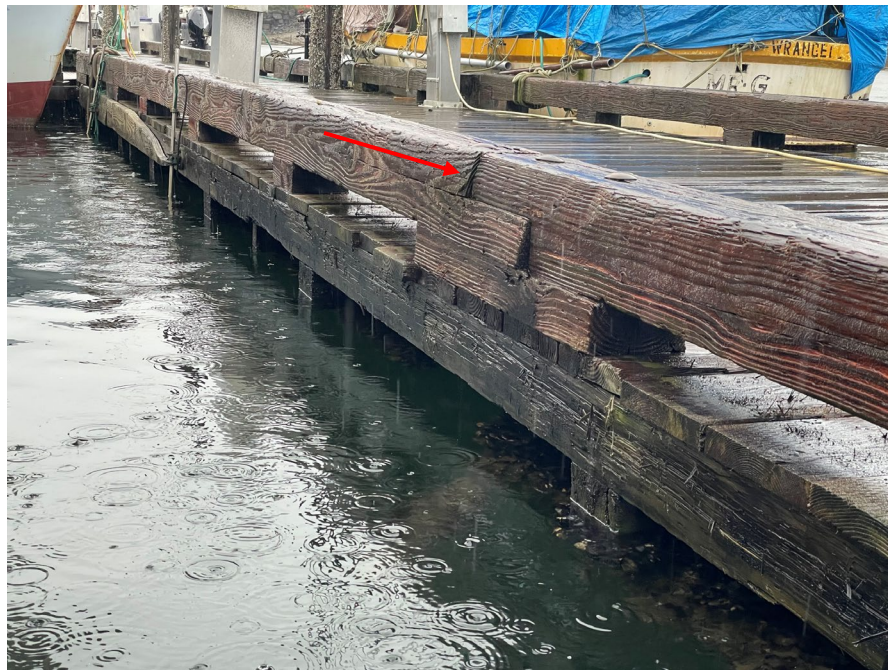
Photo 16. Damaged float to float splice connection
