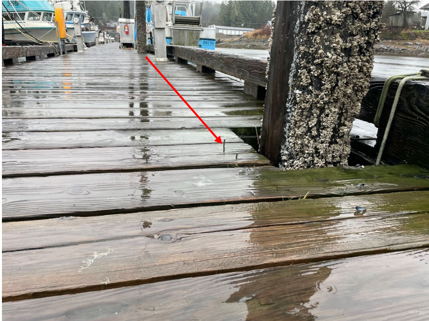
Photo 14. Several nails protruding up from decking, indicating rotten stringers beneath
