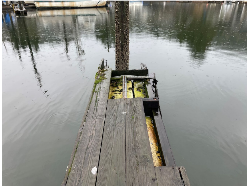
Photo 17. Significant 32' finger float damage
