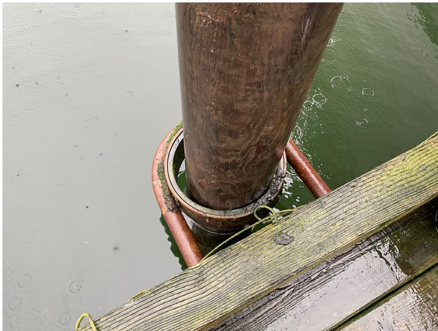
Photo 20. Corroded pile hoop
