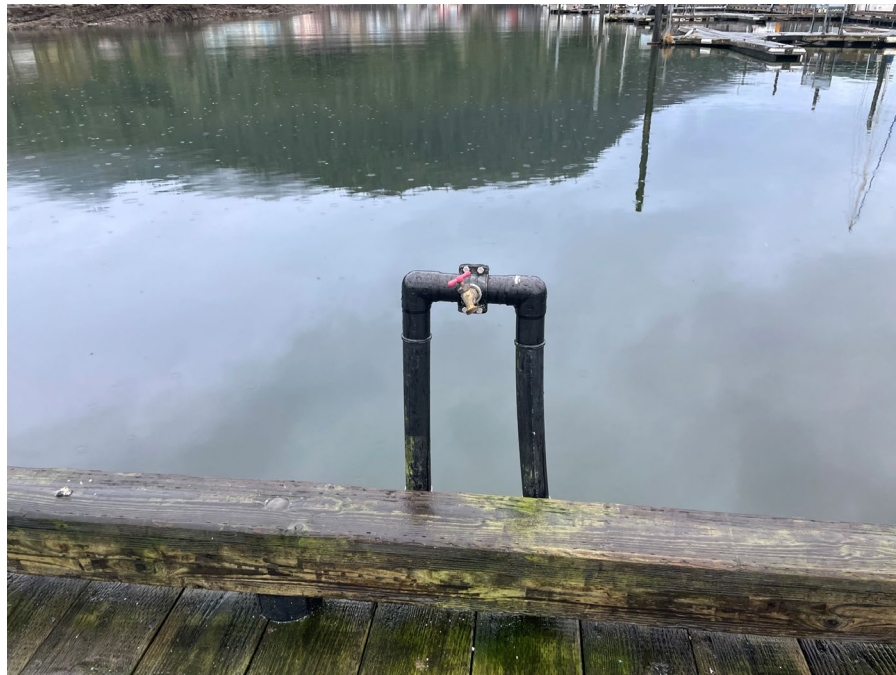
Photo 23. Typical water pedestal
