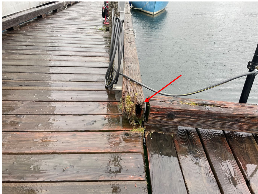
Photo 12. Typical rotten bullrail
