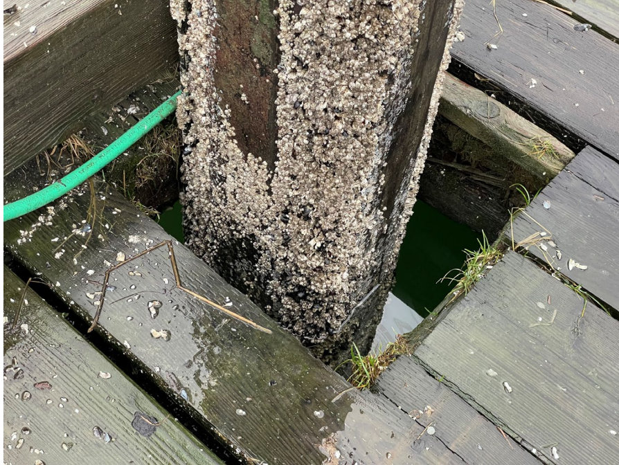
Photo 9. Worn pile/rubbing/organic growth
