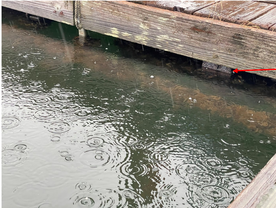
Photo 23. Submerged float timbers
