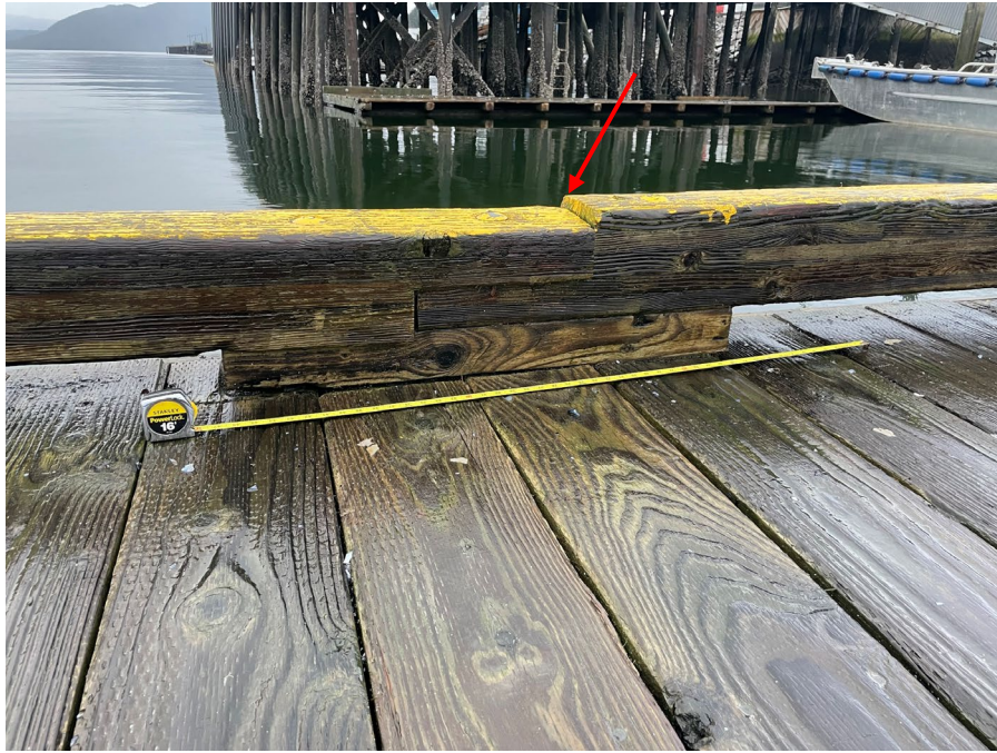
Photo 3. Damaged float to float connection splice
