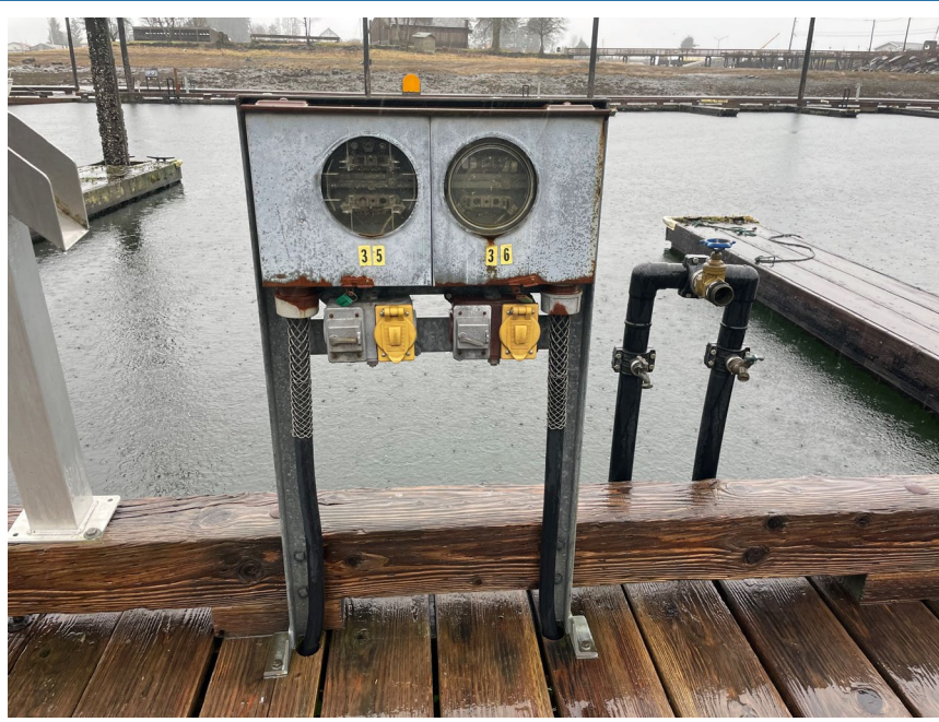
Photo 25. Typical shore power and water pedestal
