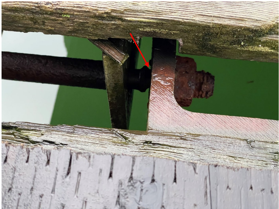
Photo 7. Typical worn/corroded mainwalk connection bolt
