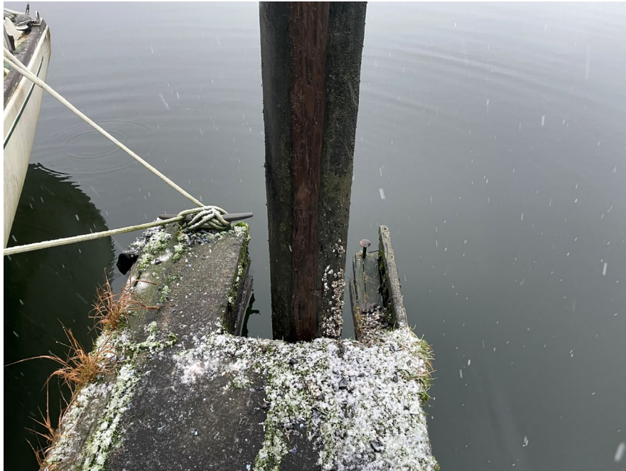
Photo 21. Damaged float/no pile restraint/rotten timbers
