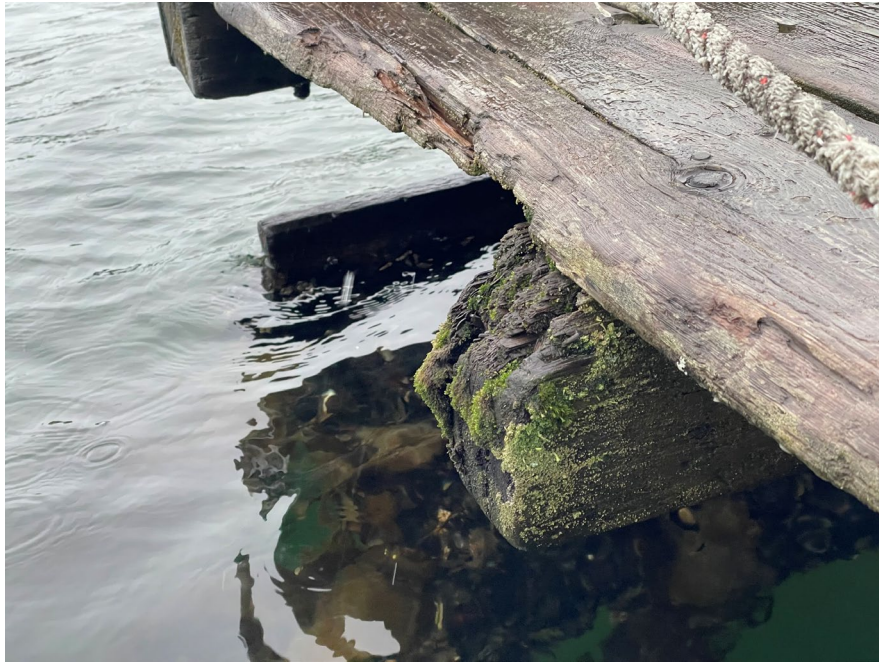
Photo 21. Rotten float stringers
