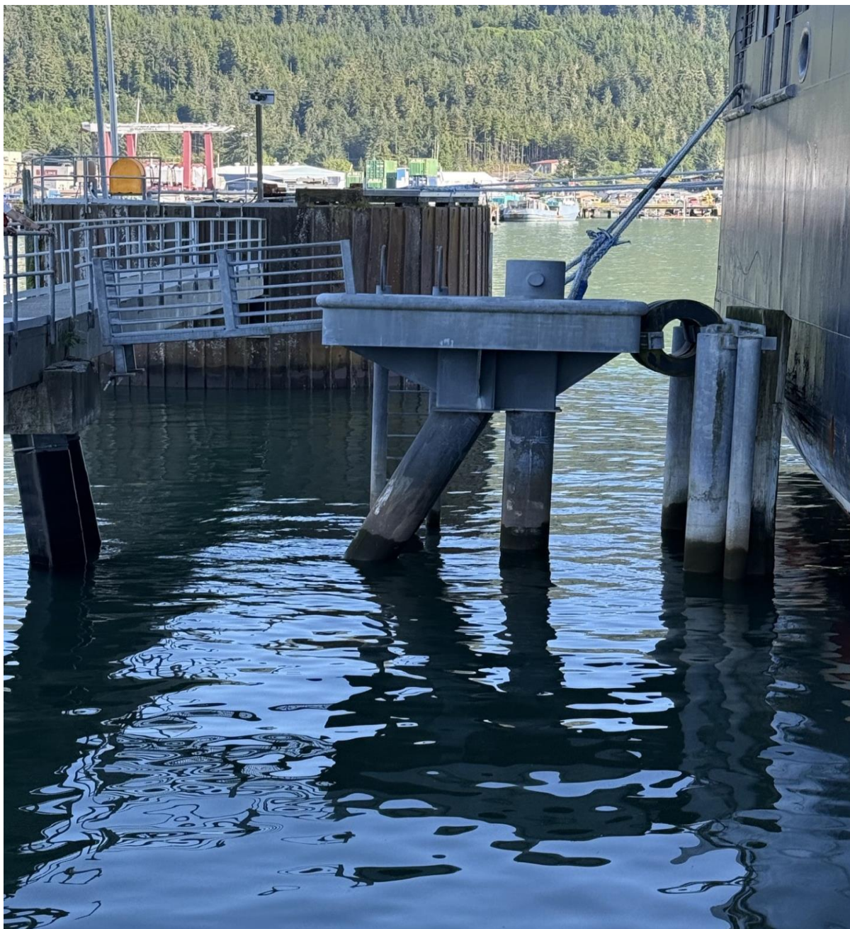
Photo 1. Overall view of the south breasting dolphin showing the visible southeast lean while the Queen Elizabeth is alongside.
