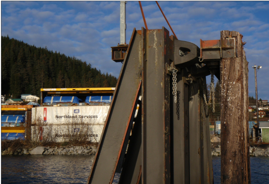
Broken stay chains at Dolphin "D".
