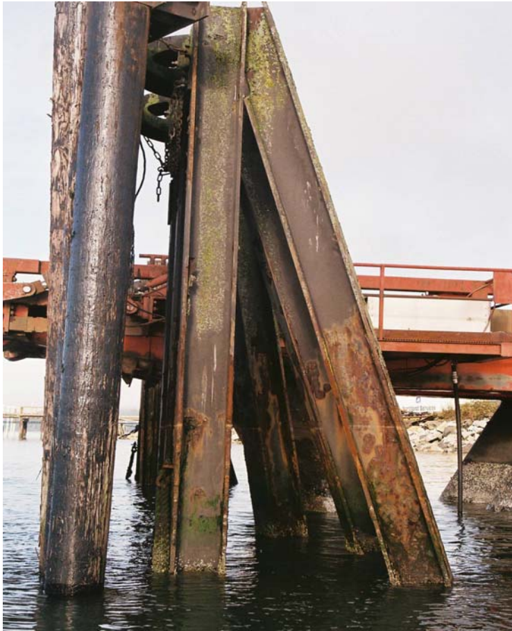
PHOTO No. 11: Breasting Dolphin F – Note the good condition of the epoxy coating at the tops of the piles and the localized coating deterioration in the splash zone. Overall these piles have been estimated to retain 75% of their coating in the combined top and splash zone.
