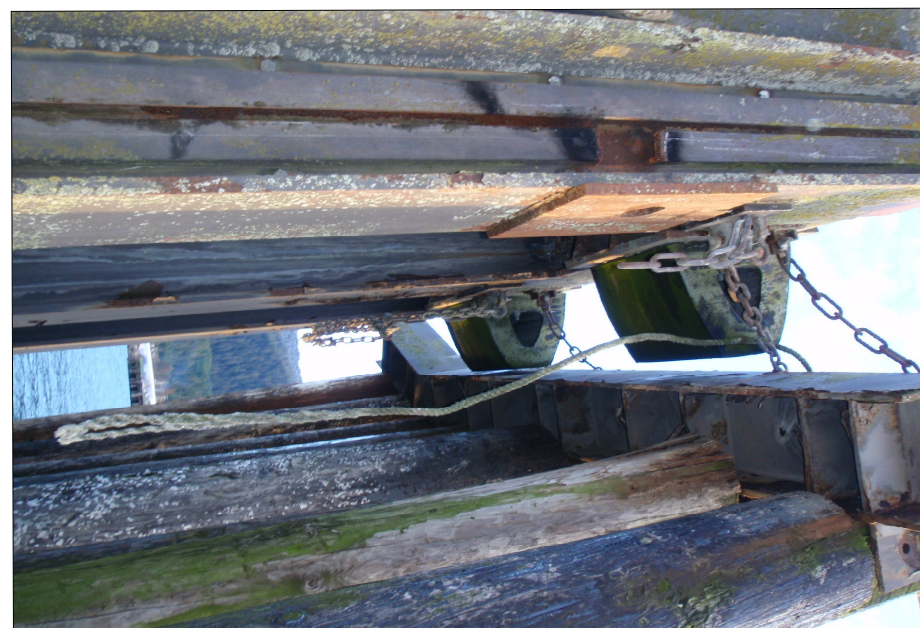
Broken stay chains at Dolphin "F".
