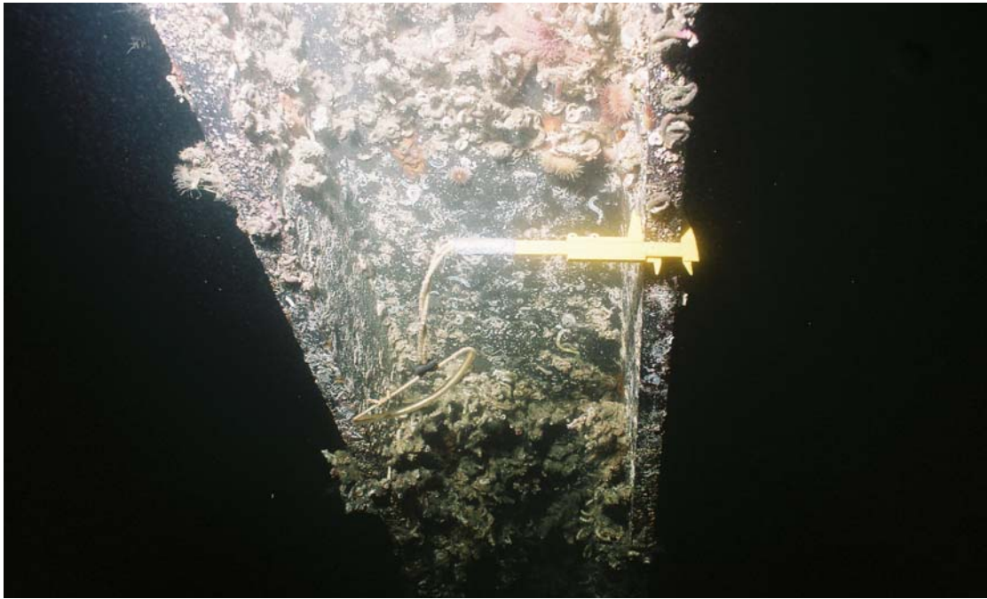
PHOTO No. 13: Breasting Dolphin C, Pile 3 Batter – Note the yellow caliper on the flange at this Level II cleaned site and the good condition of the epoxy coating in the submerged zone.
