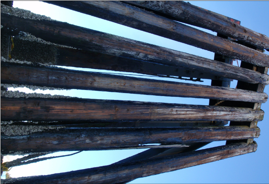
Displaced fender piles at Dolphin "D".
