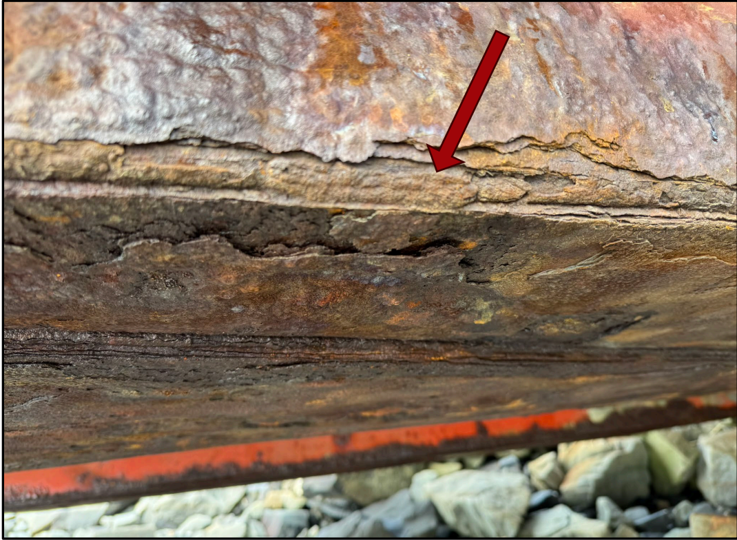
FIGURE 11. Corrosion and loss of weld material along bottom flange edge at web junction.
