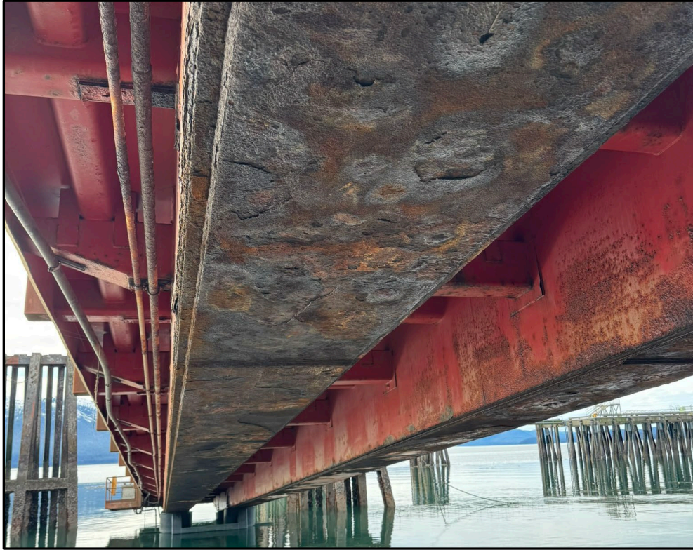
FIGURE 9. Typical barge ramp girder bottom flange – coating loss and laminar corrosion.
