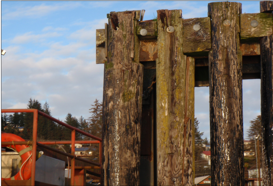
Broken fender pile at Dolphin "F".
