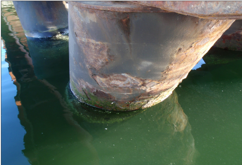
Typical coating failing/minor corrosion of ramp tank support strut.
