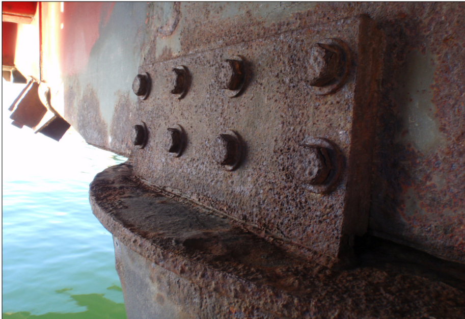
Coating failure/corrosion at ramp/support tank connection assemblies.
