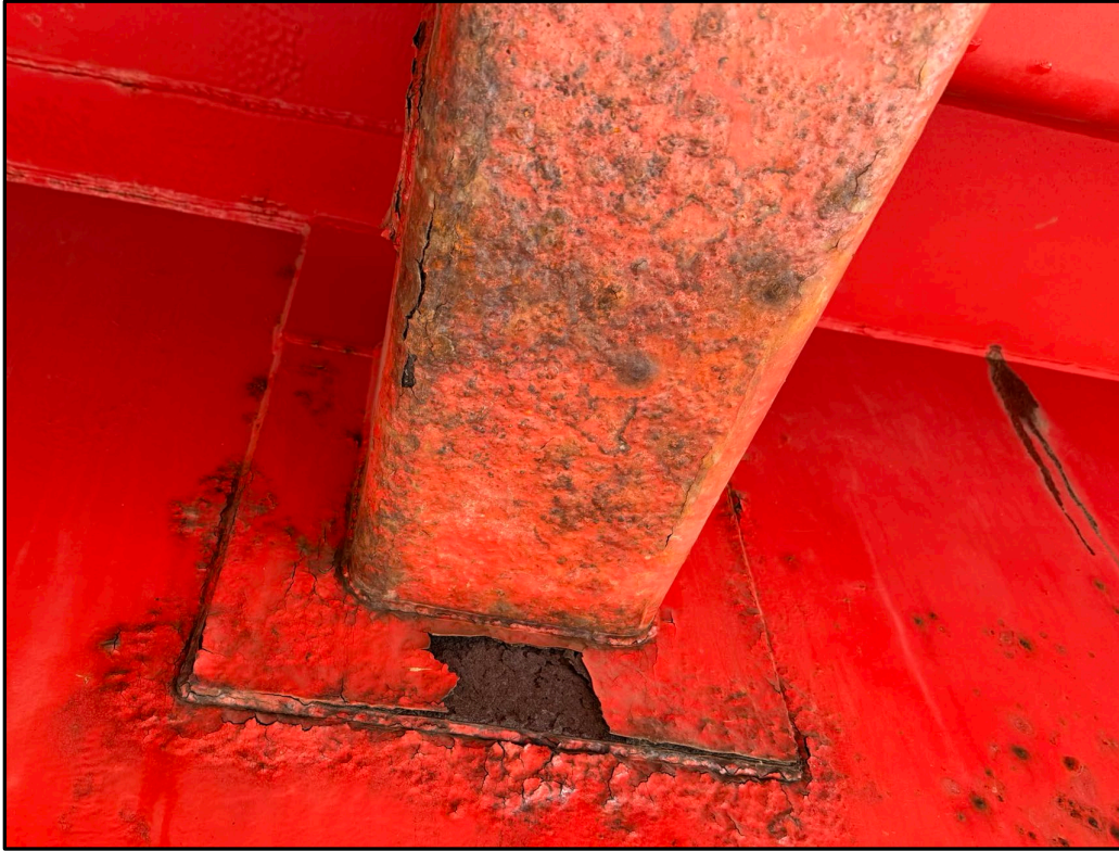
FIGURE 15. Close-up of advanced corrosion at typical floor beam connection.
