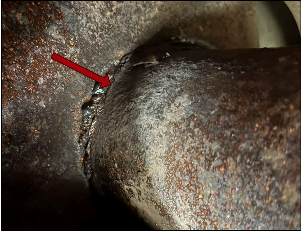
FIGURE 13. Cracked repair weld at abutment bearing pivot pipe.
