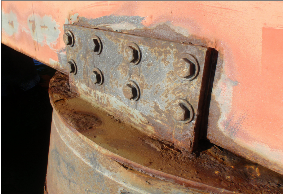
Coating failure/corrosion at ramp/support tank connection assemblies.
