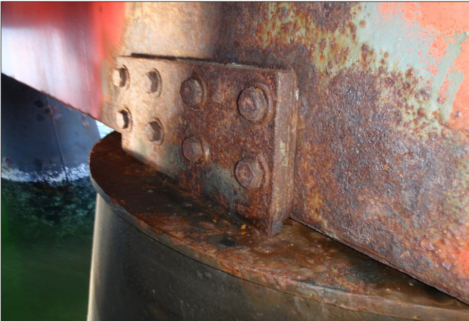
Coating failure/corrosion at ramp/support tank connection assemblies.
