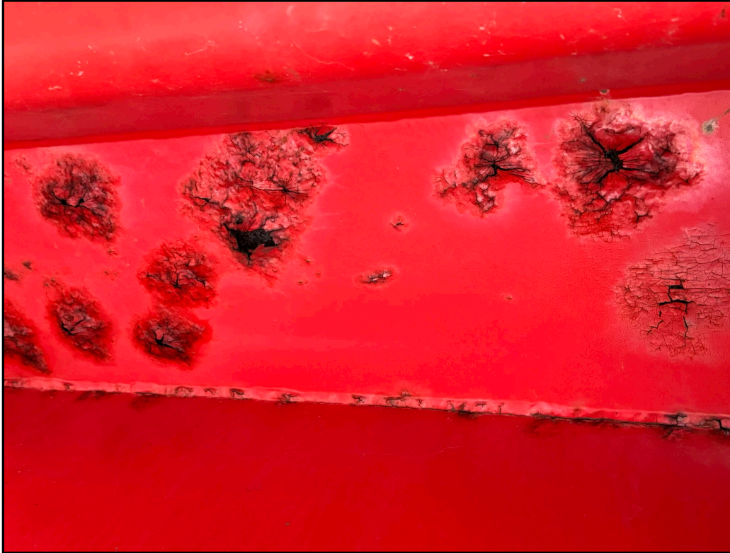
FIGURE 16. Typical blistering of deck plate (underside) between deck ribs.
