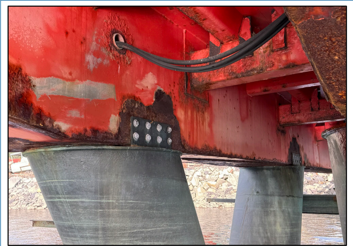
FIGURE 5. Flotation tank connection plates with new bolts.
