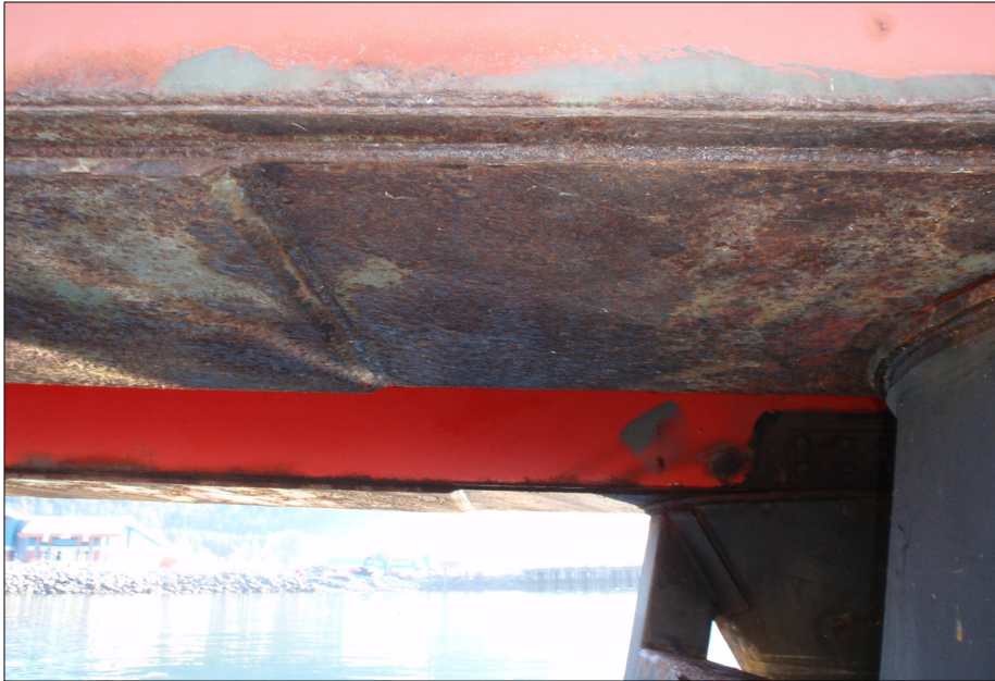
Typical minor corrosion of ramp girder bottom flange.
