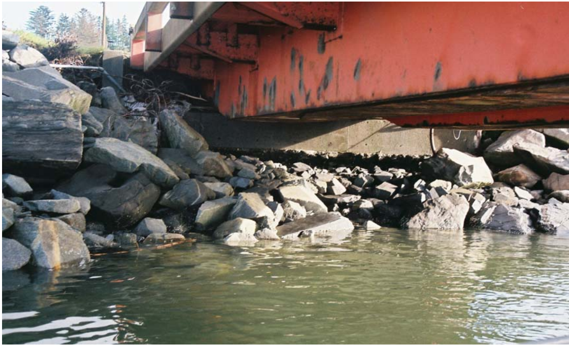
PHOTO No. 3: Transfer Span Bridge Seat – Note the undermining of the concrete bridge seat. Also note the localized failure of the painted coating on the transfer span members.
