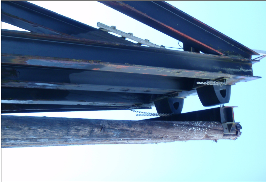
Broken stay chains at Dolphin "D".
