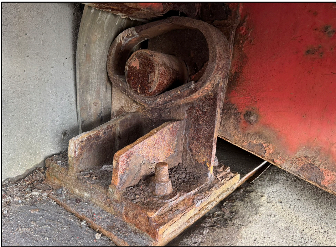
FIGURE 12. Corrosion at abutment bearing assembly; deformed/repairs saddle bearing.
