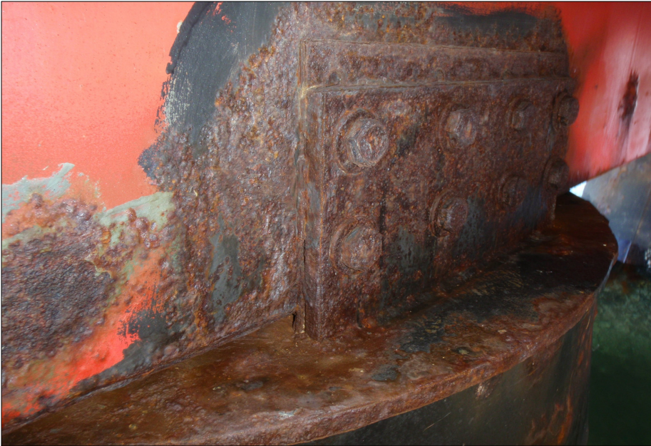
Coating failure/corrosion at ramp/support tank connection assemblies.
