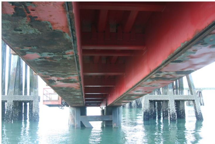
Figure 3 - coating failure along the barge ramp girder soffits
