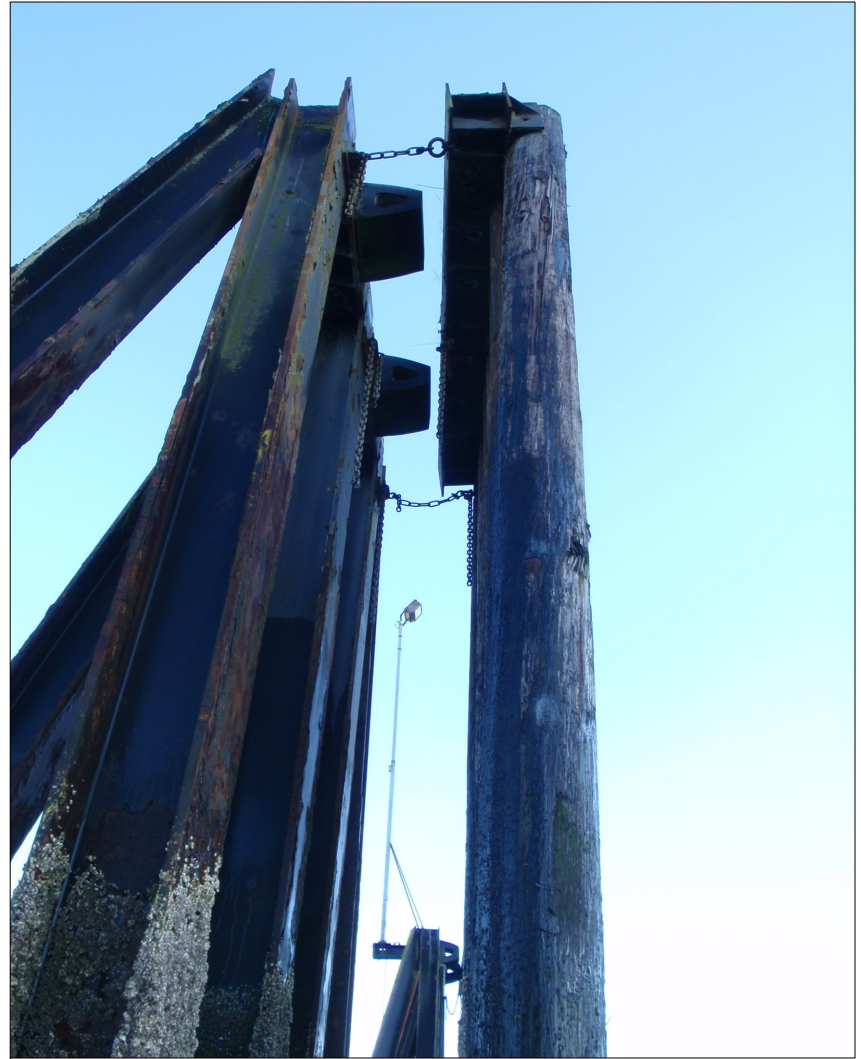
Broken stay chains at Dolphin "C".
