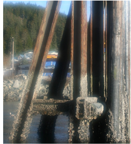
Figure 2 - coating failure in the splash zone
