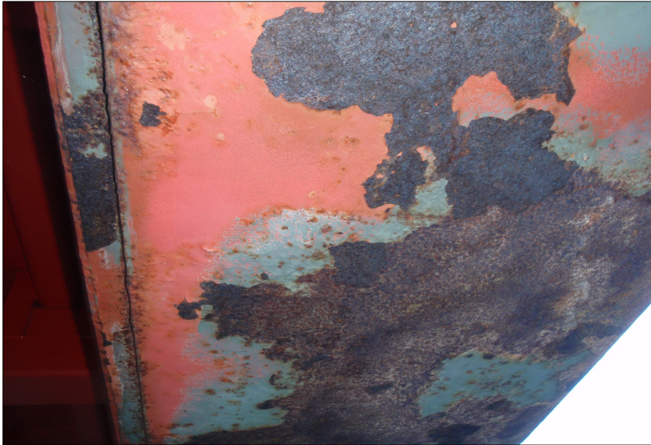
Typical coating failure/corrosion of girder bottom flange.
