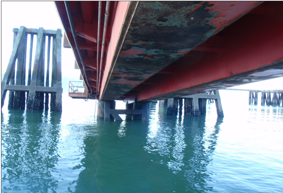
54 Ramp box-girder bottom flanges; coating failure, minor corrosion, typical.
