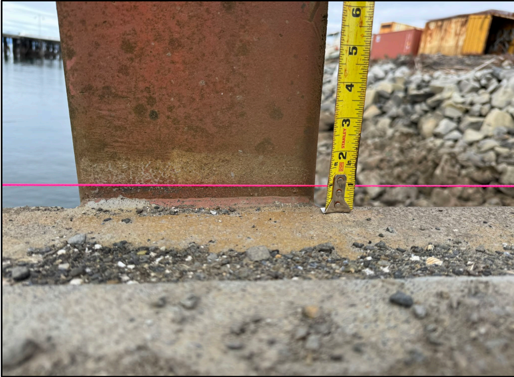
FIGURE 17. Sag at mid-span of the barge ramp (i.e. ramp bent due to overloading).
