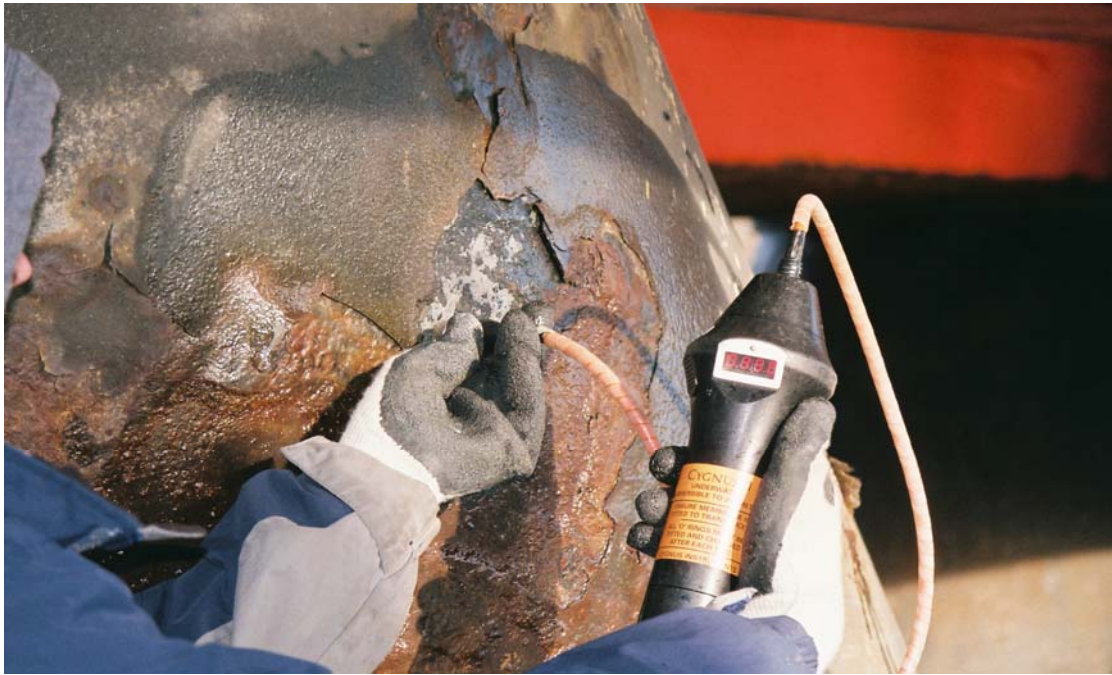
PHOTO No. 5: Southern Floatation Tank Pipe Strut – Note the coating failure and corrosive scale evident in the splash zone. Level III ultrasonic thickness measurements found the remaining thickness to be 0.357 inches.
