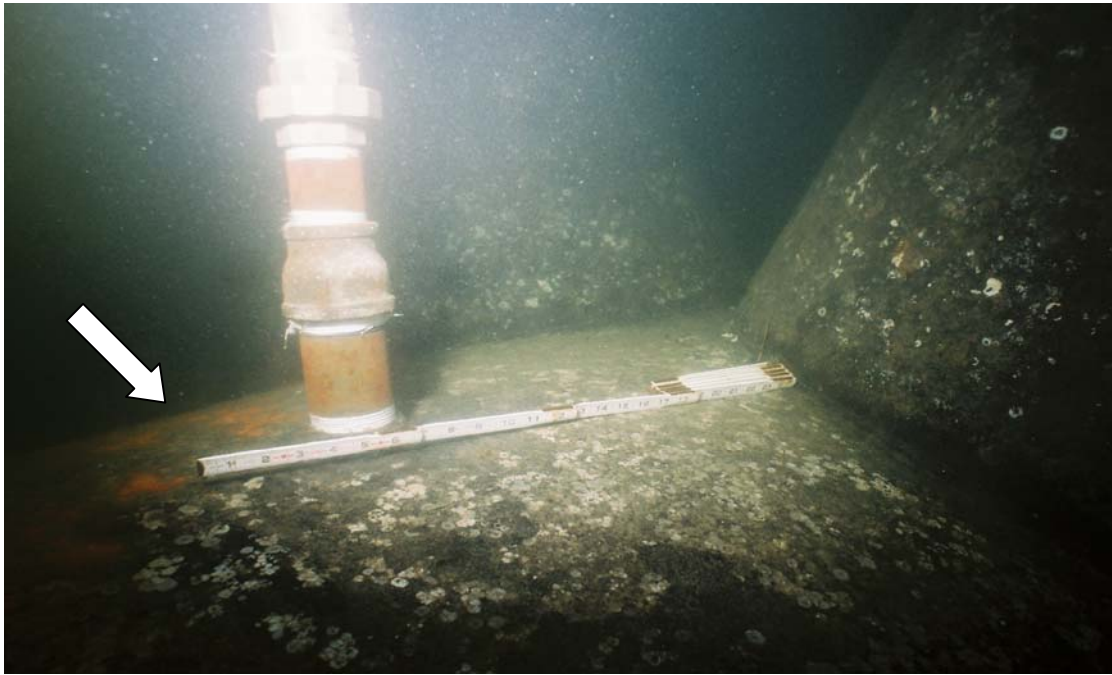
PHOTO No. 7: Floatation Tank, Air Inlet Port – Note the good condition of the air inlet port located at the south end at the crown of the 9 ft. dia. tank. Also note the good condition of the coating on the two pipe struts and the minor coating deterioration in the vicinity of the inlet.
