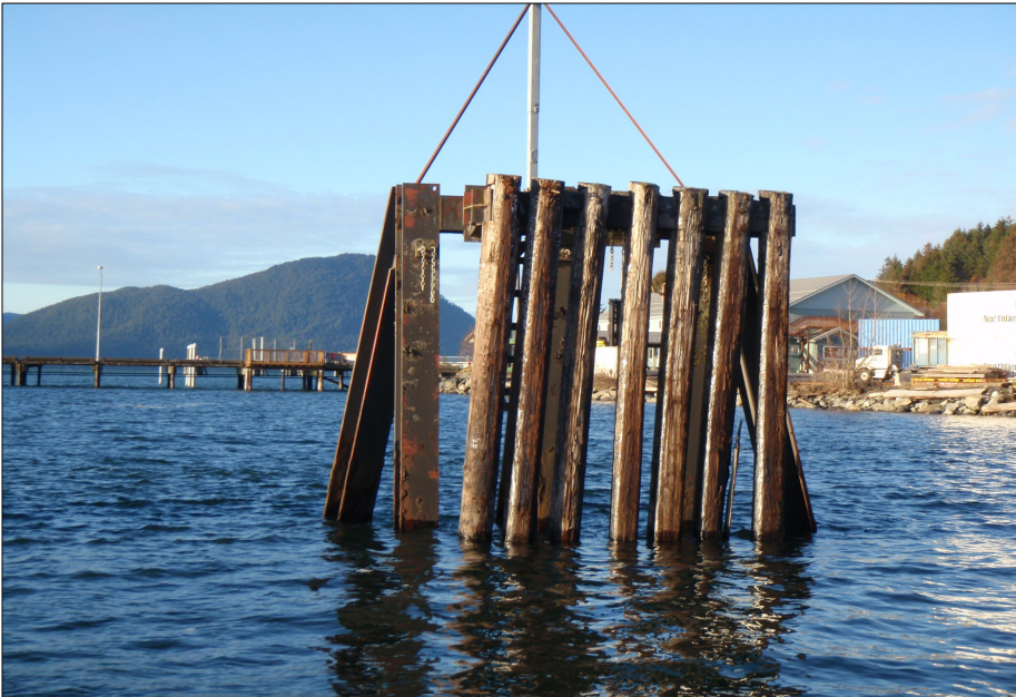
Displaced fender piles at Dolphin "D", looking north.
