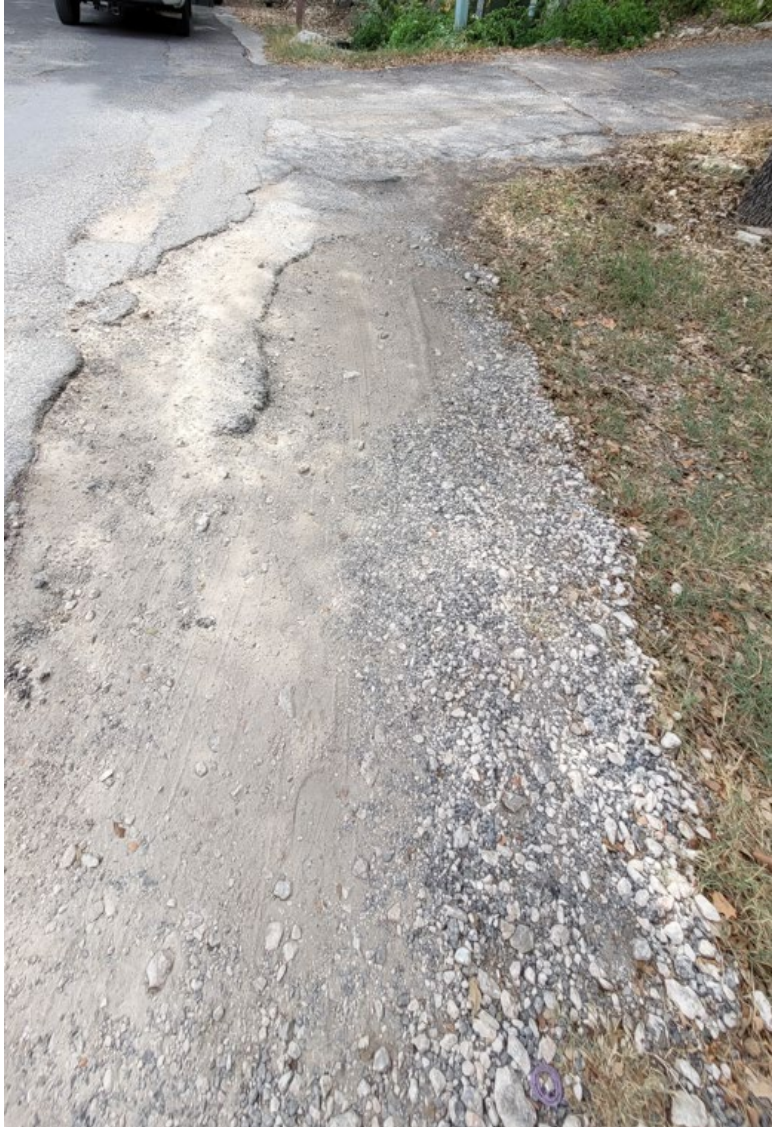
4 Tremont Trace – Before (Asphalt Driveway & Approach)
