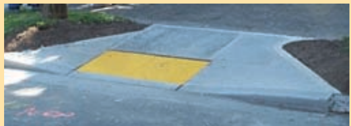
An example of a jurisdictional change is a city-wide policy for the installation of ADA-compliant curb ramps.
