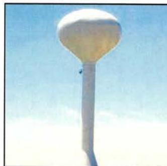
Winnebago's potable water system utilizes a water tower for storage. The tower is located at Main Street and Church Street.
