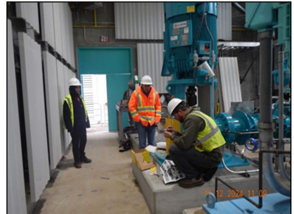
Inspection and testing a new finished water pump at WTP
