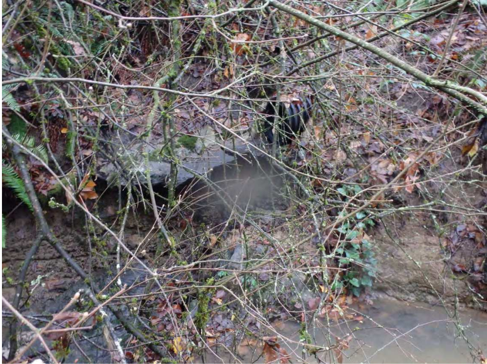
Photo 16 Perched Culvert on Right Bank
