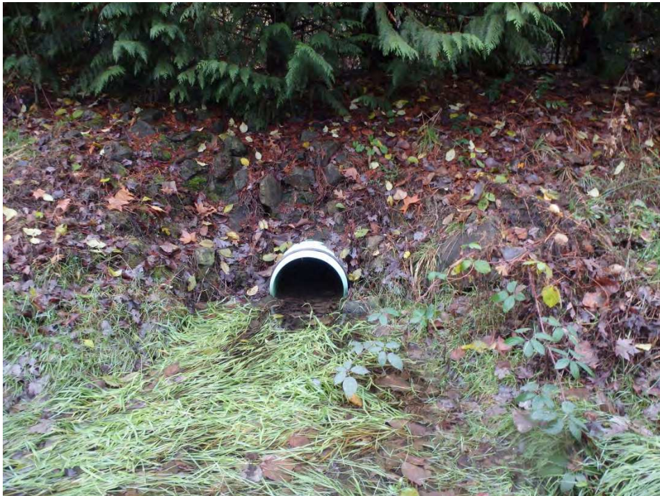
Photo 6 Partly submerged 18-inch CCP contributing culvert
