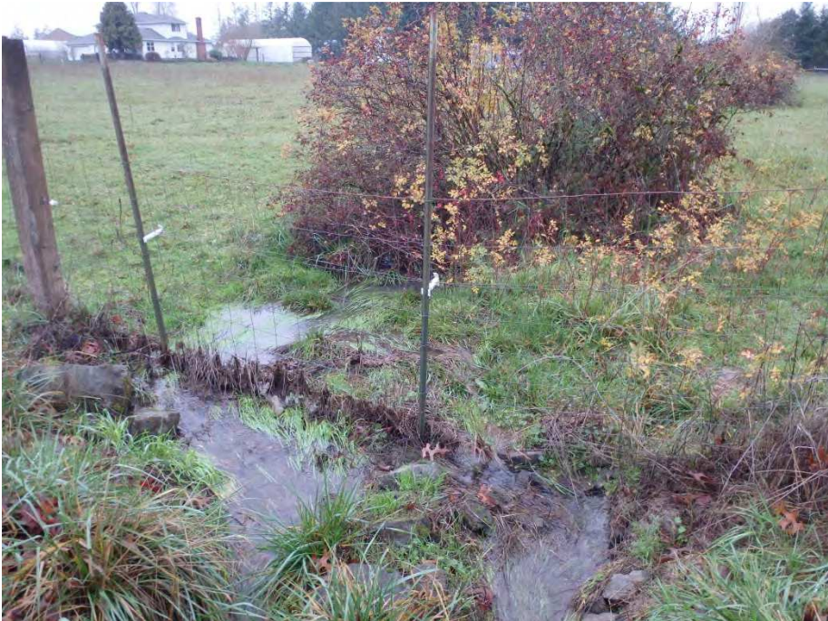
Photo 1 Channel in ROW on Frog Property
