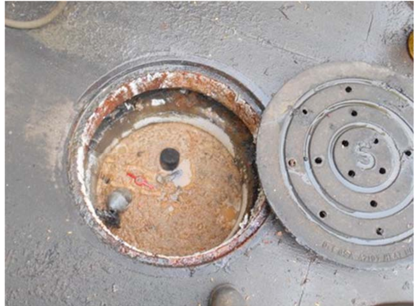
Grease in manhole
