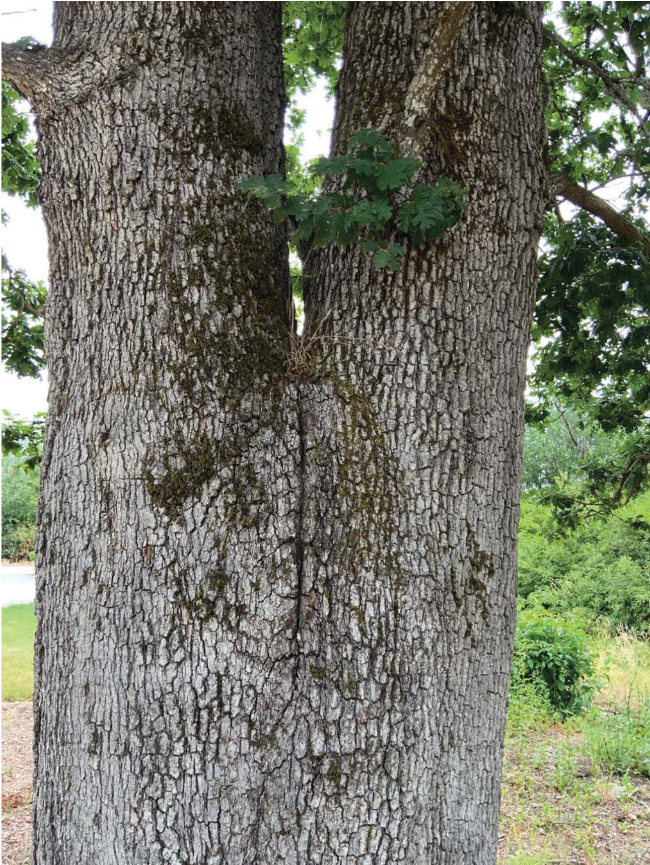
Photo 12. Tree #57630 - Codominant stems with included bark. Morgan believes she has observed a squirrel crawling into this juncture in the past, indicating that the cavity between the stems is much larger than it would seem from the outside. Recommend installing a brace and cables.
