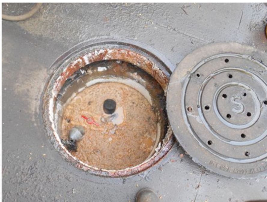
Grease in manhole
