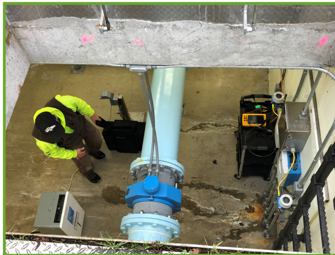
Measuring flow with ultrasonic flowmeter
