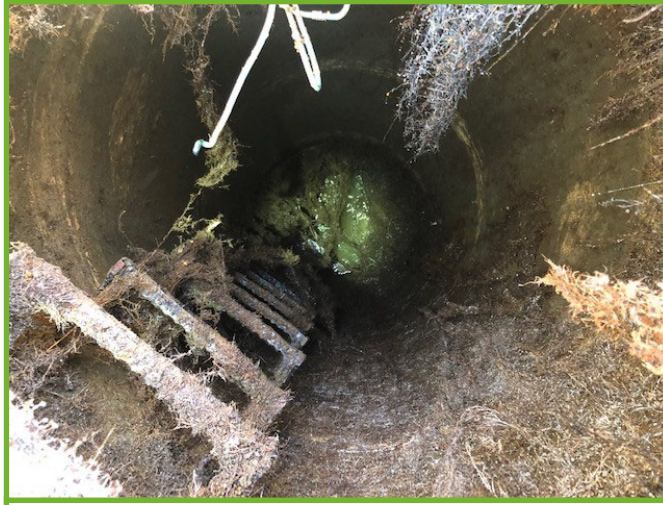
Roots draping in a manhole
