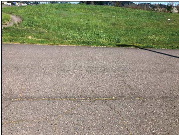
Photo 1: North Entrance Drive – Fatigue Cracking
