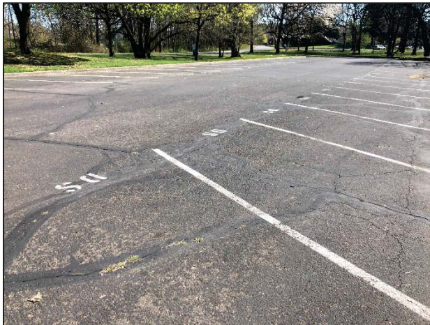
Photo 3: North Parking Bay –Random/ Transverse/ Longitudinal Cracking
