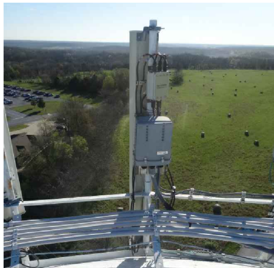
4 EXISTING ALPHA SECTOR RRU AND RAYCAP LOCATION N.T.S.
