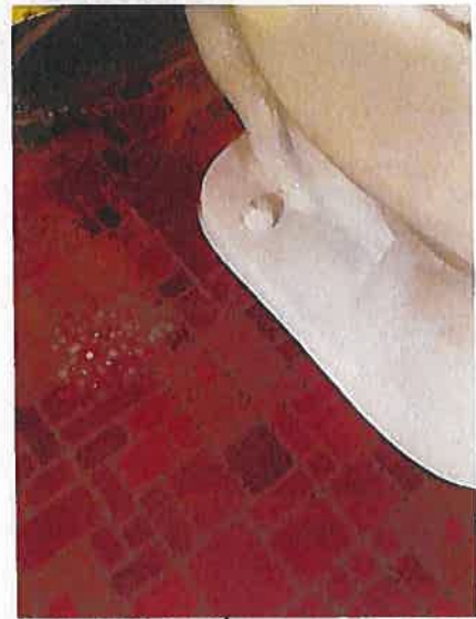
Past repairs noted
