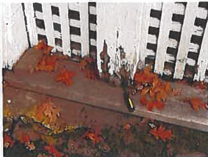
Northeast Side- Post floating and damaged
