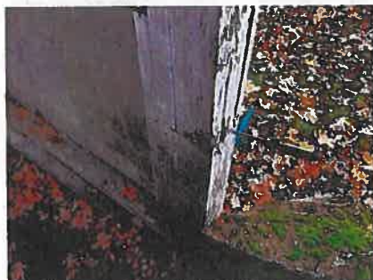
Southwest corner Wood Decay
