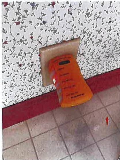
Non grounded outlet near the tub below the window-
