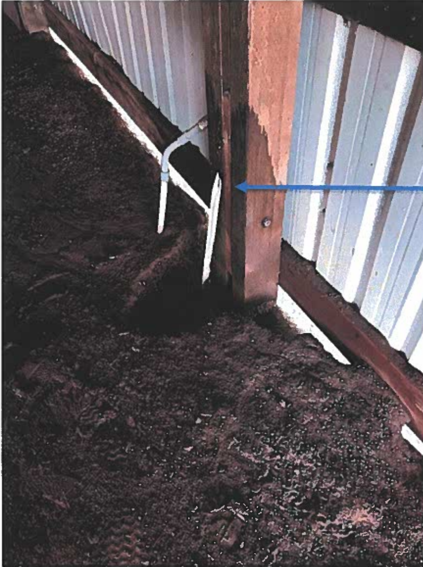
Broken waterline before repair
