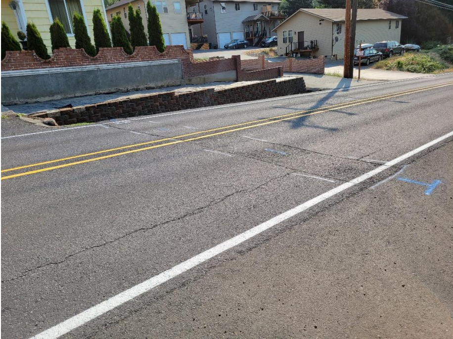
Photograph 3: 612/614 E. Jewett Blvd Service Line
