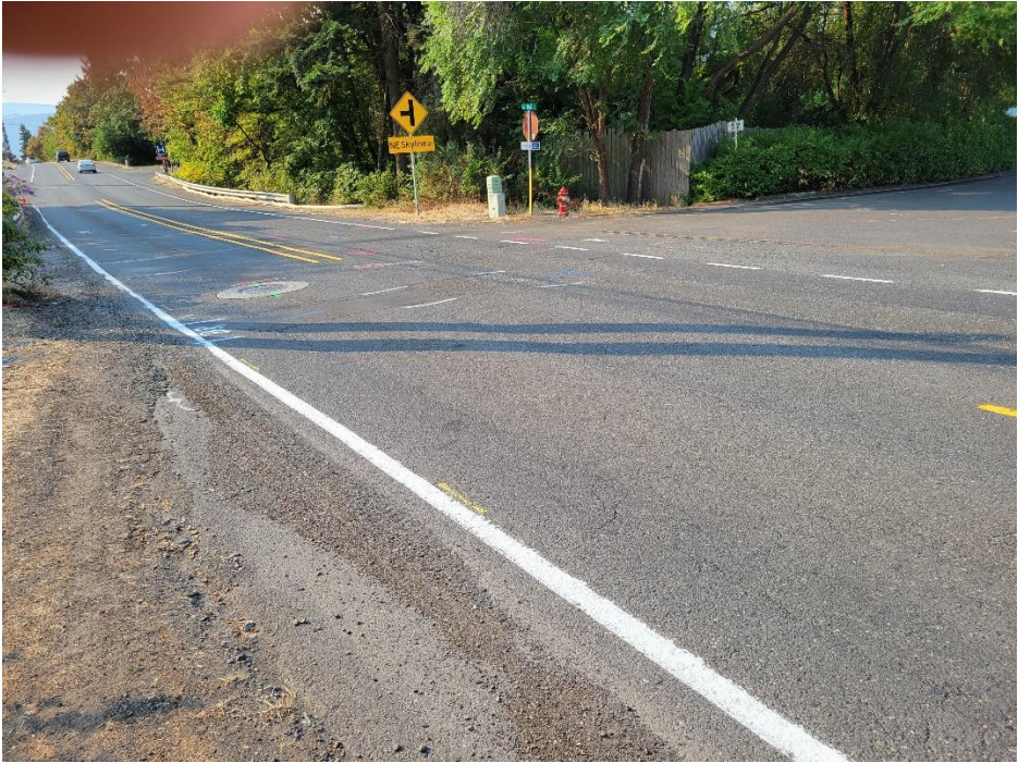
Photograph 6: 850 E. Jewett Blvd Service Line
