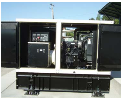
Northshore Utility District – Lift Station 4 Generator
