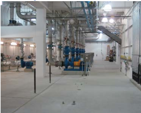
Lake Stevens Sewer District – Permeate Pumps
