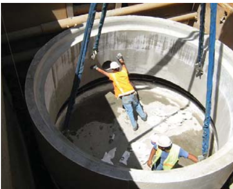
Bothell – Lift Station 2 Wet Well
