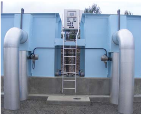
Castle Rock – Addition of Upflow Clarifiers
