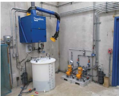
Naval Base Kitsap (Bangor) – Fluoridation Facility
