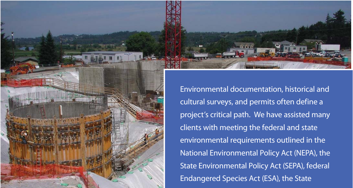
Lake Stevens Sewer District – Sunnyside Wastewater Treatment Facility
