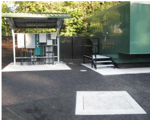
Silver Lake Water & Sewer District – Valmont Generator and Electrical Rack
