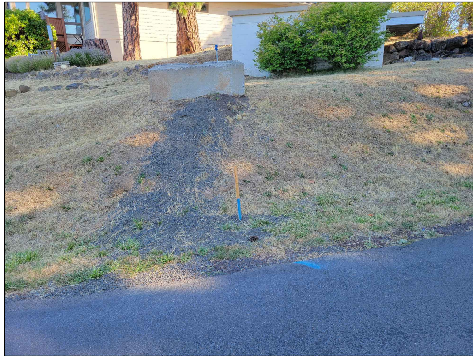
P1 C-101 6" CONNECTION WITH TEE LOCATION VIEW TO NORTHWEST NTS
