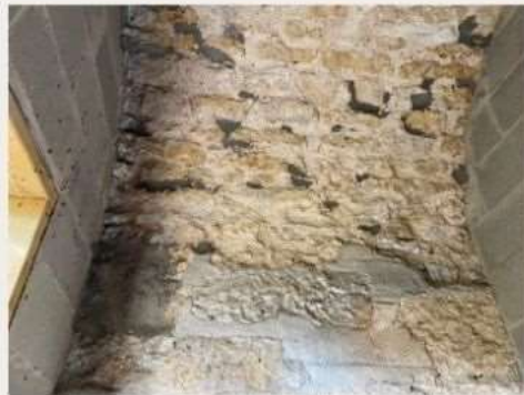
Mortar Joint Deterioration
