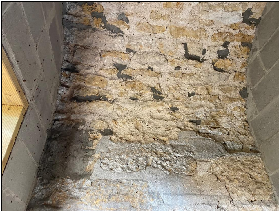
Photo 25: Different mortar at entry arch
