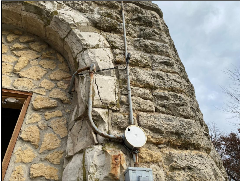
Photo 22: Cracked stone in entryway arch
