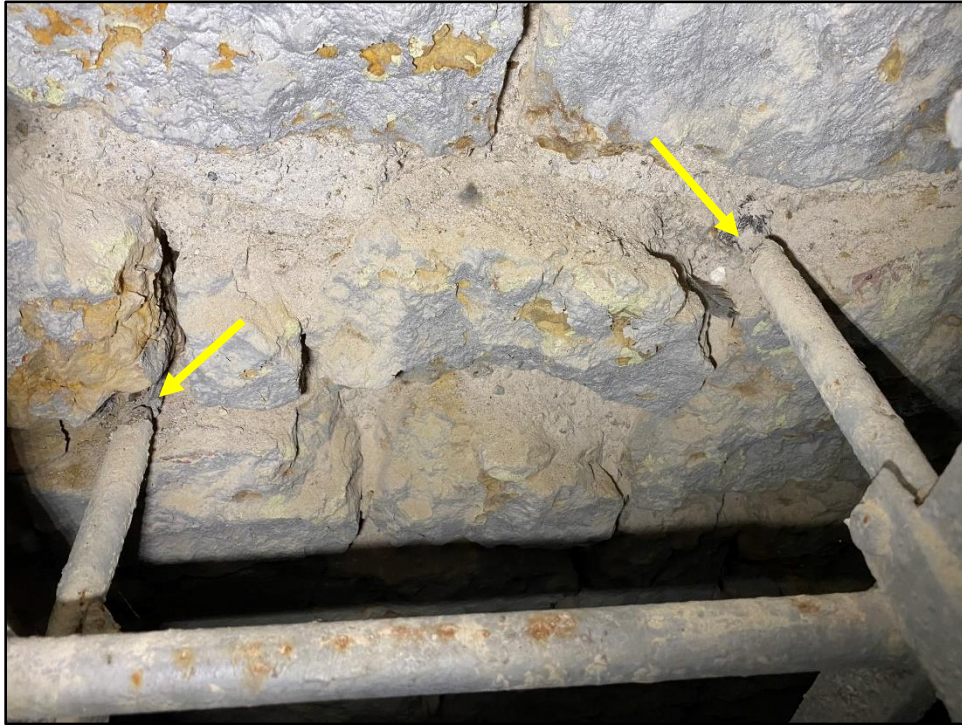
Photo 37: Corroded ladder connections at wall
