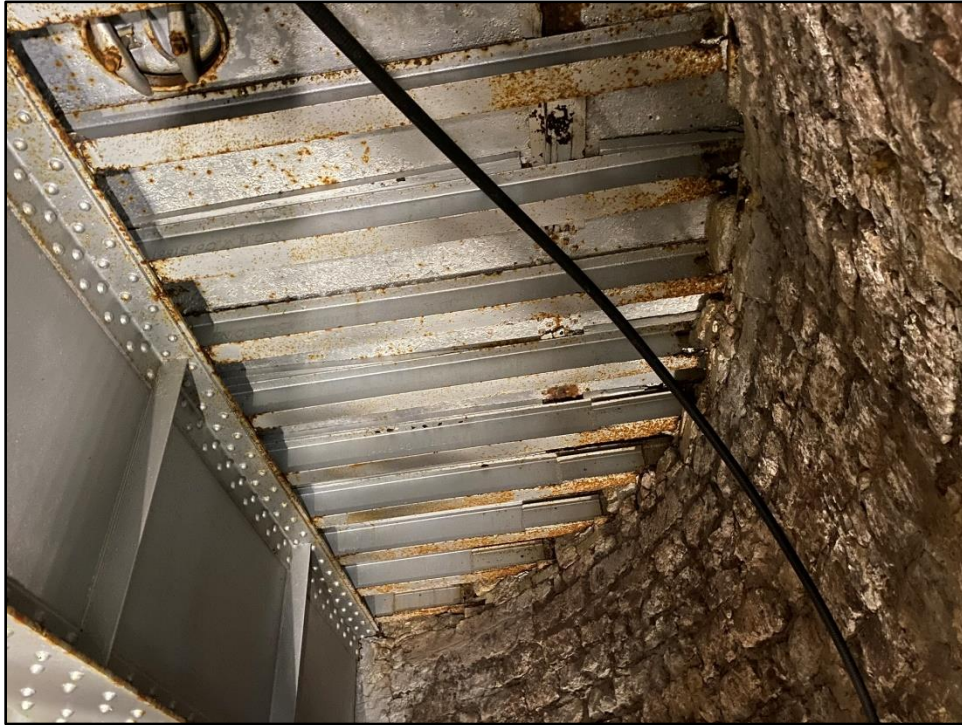
Photo 33: General surface corrosion of tank support beams with an increase near walls
