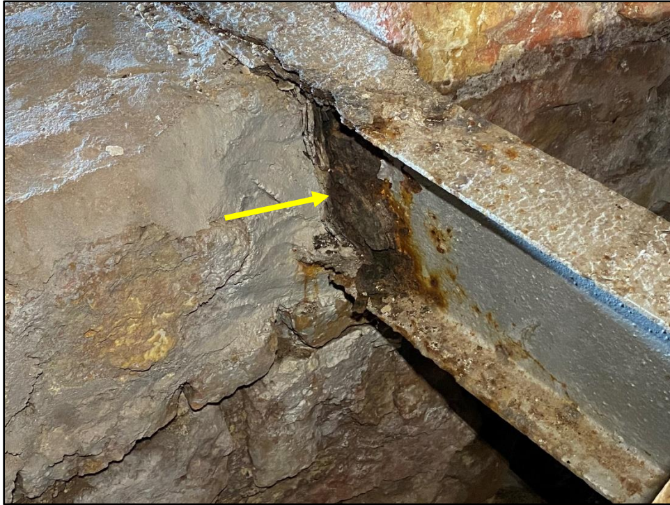
Photo 35: Corroding floor beam at exit to exterior platform
