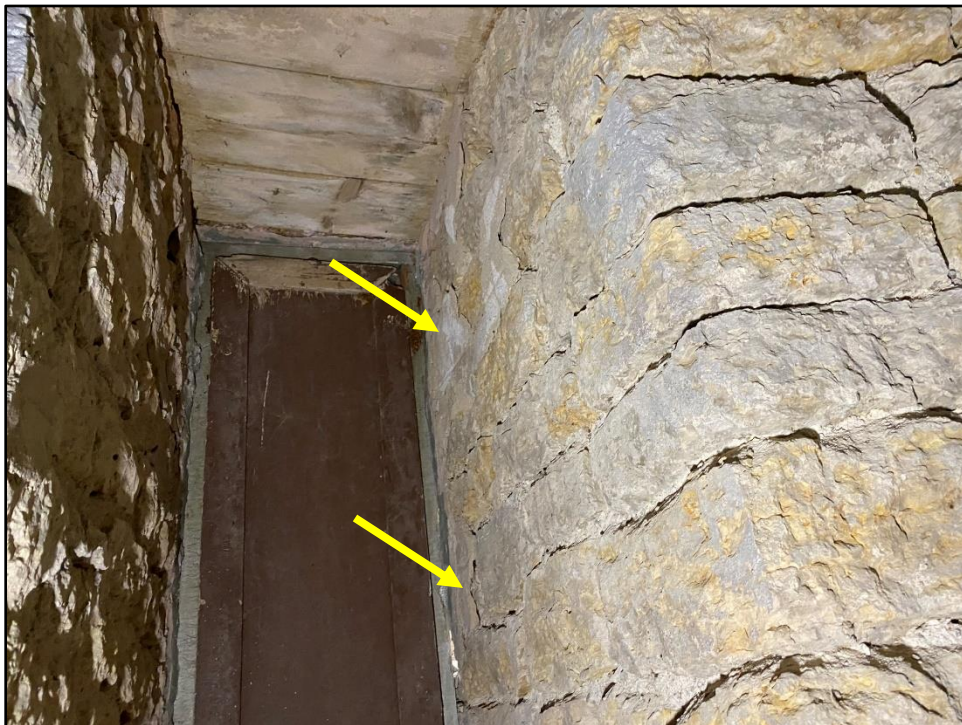
Photo 19: Spalled stone on "door" walls
