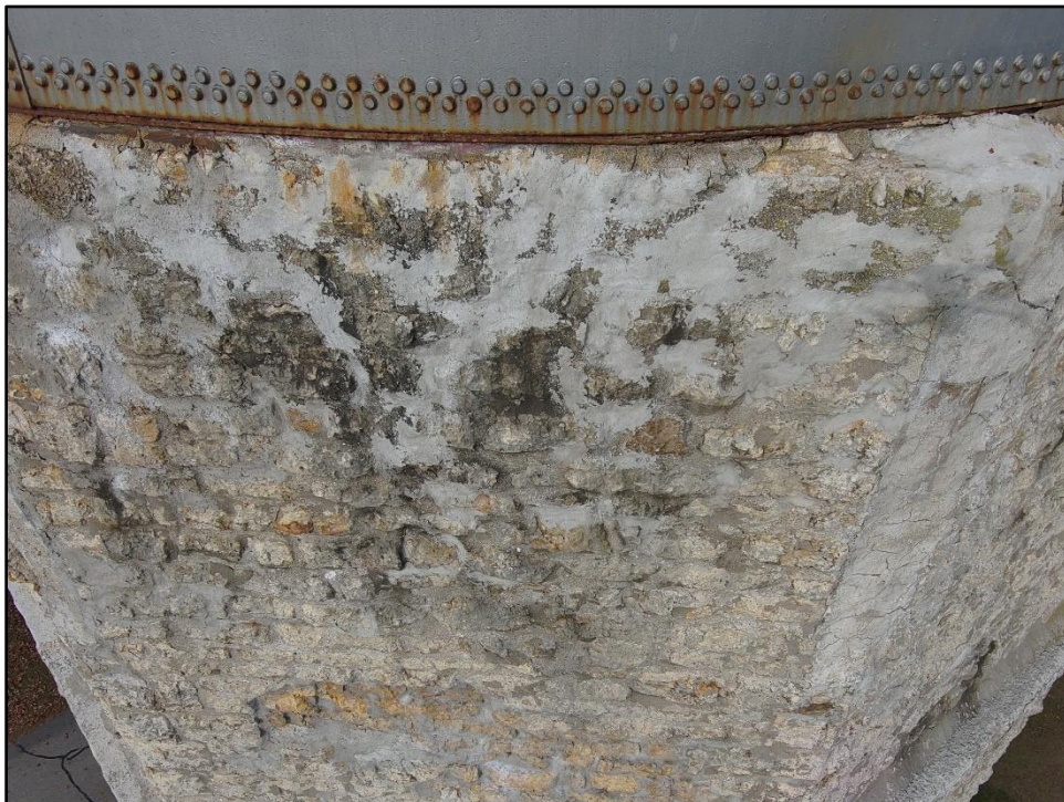
Photo 27: Repointing mortar at top of tower
