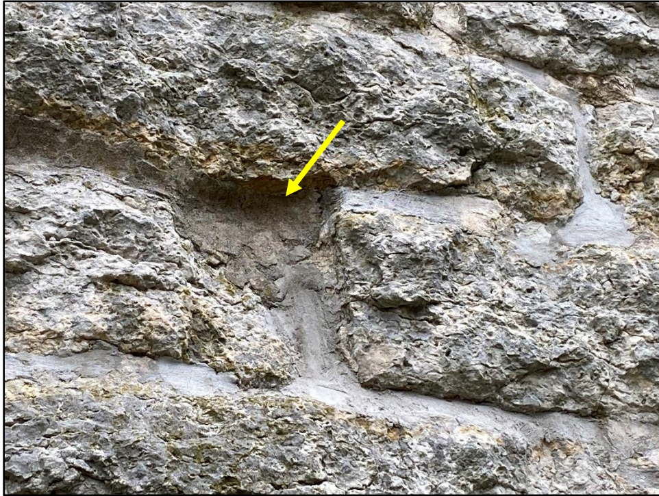
Photo 18: Isolated locations of stone spalls
