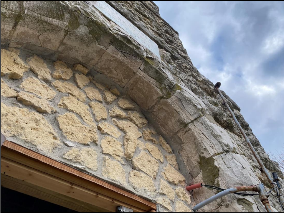
Photo 23: Cracked stone in entryway arch
