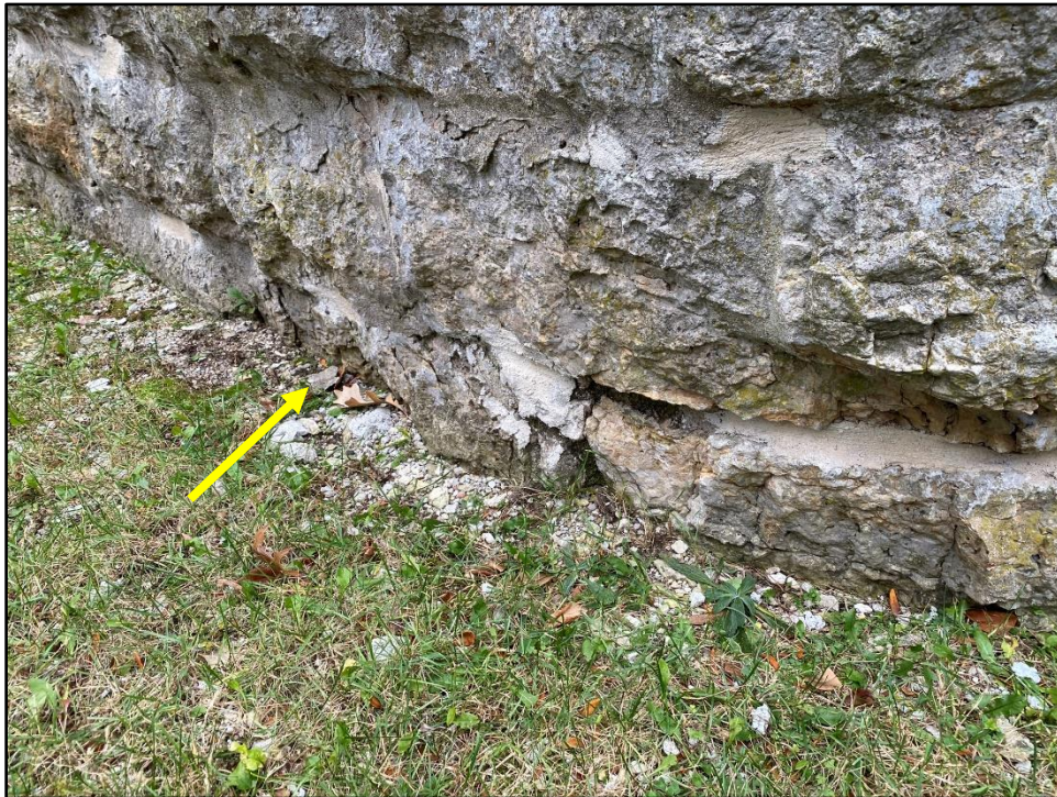
Photo 21: Stone deterioration at base of wall
