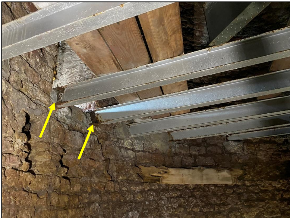
Photo 34: Signs of floor beam corrosion at walls
