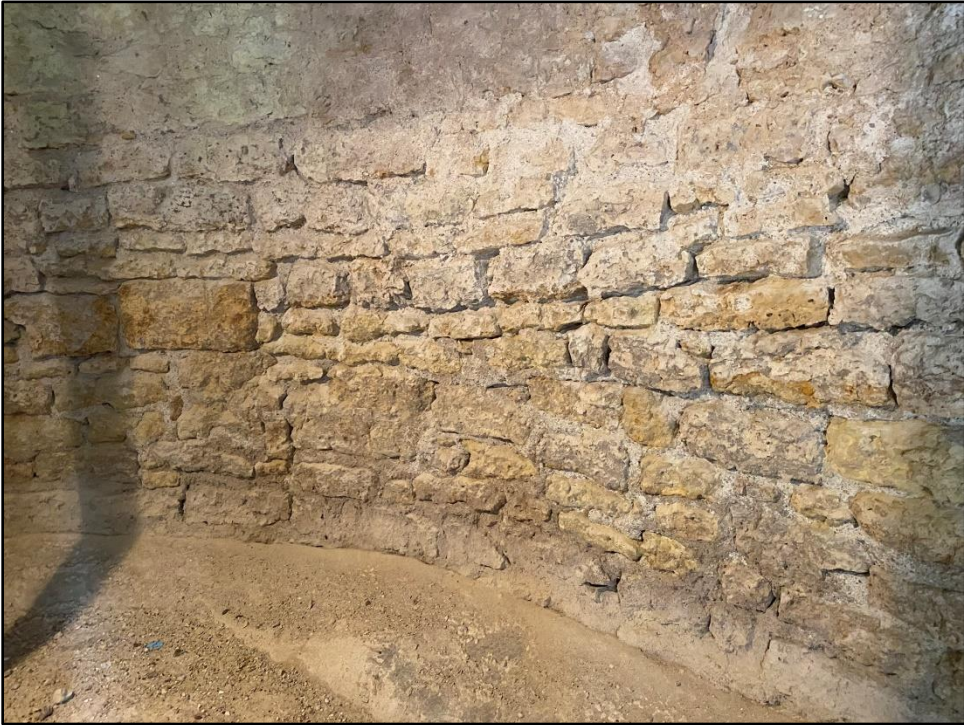
Photo 28: Deteriorated joints on interior – dust on floor is deteriorated mortar
