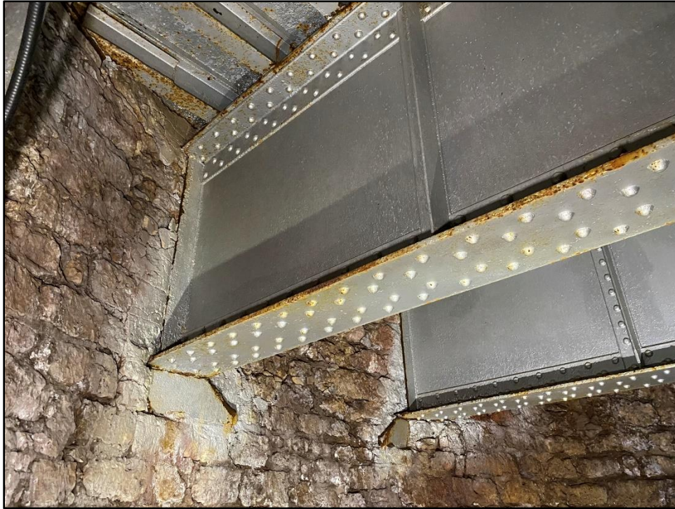
Photo 31: General light corrosion on support structure
