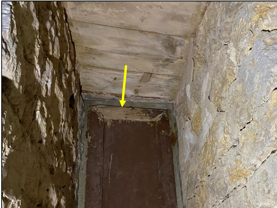
Photo 39: Minor wood deterioration at access panels
