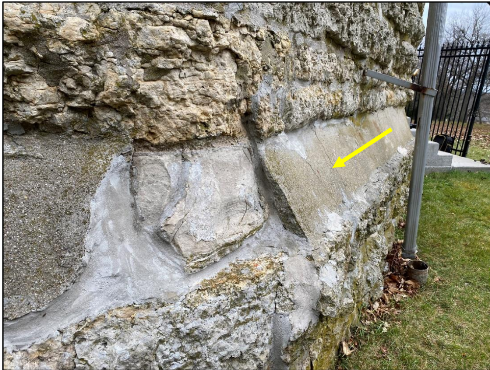
Photo 30: Cracked and missing concrete/mortar wash
