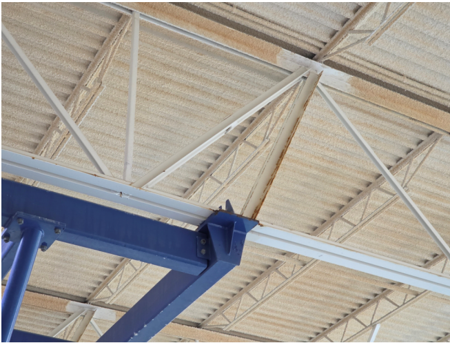
15. CORROSION ON ROOF/CEILING SYSTEM
