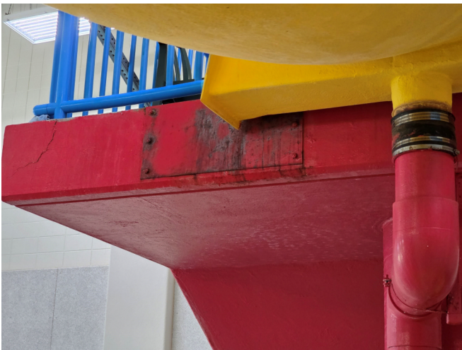
11. CORROSION ON METAL PLATE UNDER STARTING TUB
