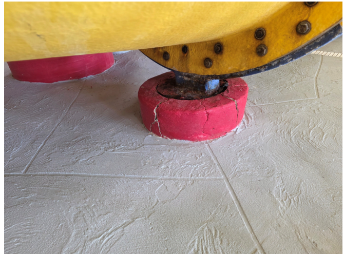
18. CRACKED PEDESTAL AND CORRODED SUPPORT PLATE
