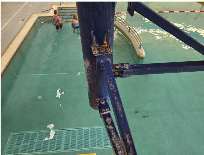
5. FLAKING/WORE PAINT AND FINISH
