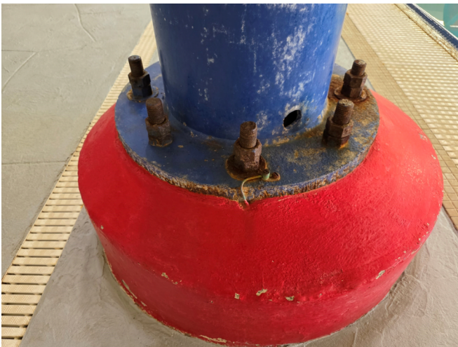
17. CORROSION ON SUPPORT TREE FLANGE AND FASTENERS
