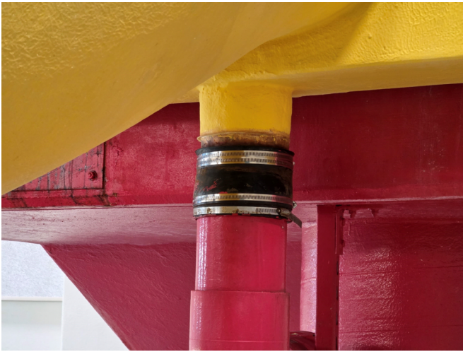
19. MINOR CORROSION ON SLIDE SUPPLY COUPLING
