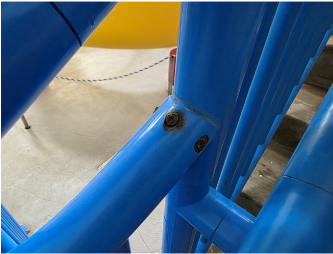
3. CORROSION ON FASTENERS
