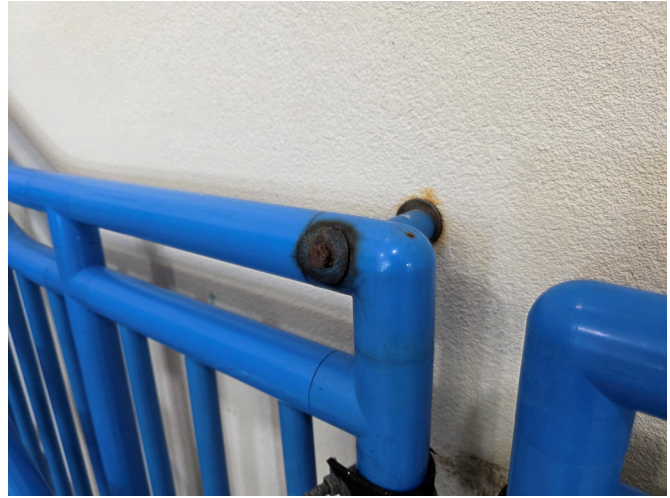
2. CORROSION ON FASTENERS
