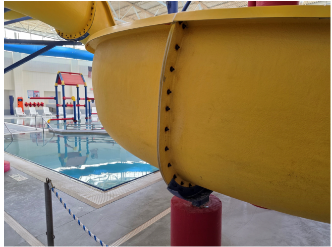
4. CORROSION ON FASTENERS
