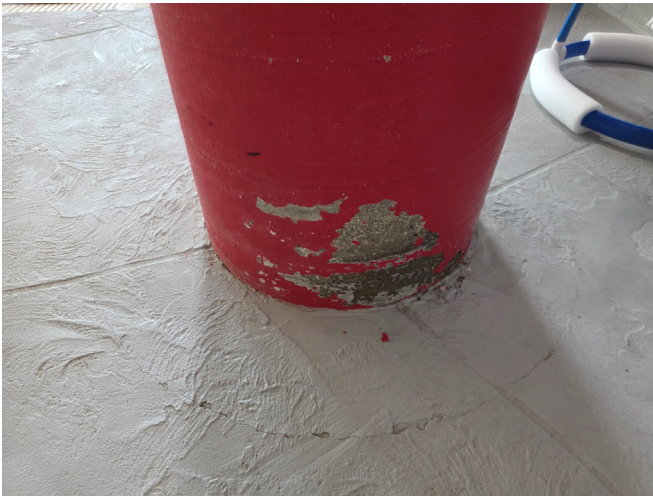
7. FLAKING/WORE PAINT AND FINISH
