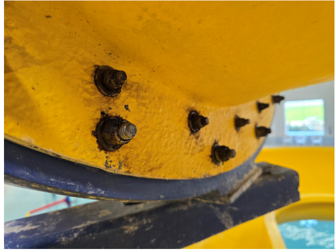
20. MISSING THREAD CAPS
