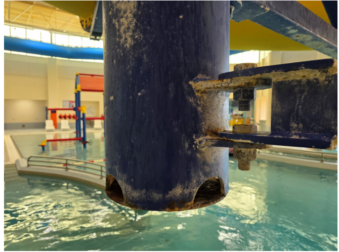
14. CORROSION AND PAINT WEAR ON SLIDE SUPPORT TREE
