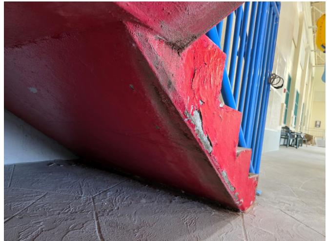
6. FLAKING/WORE PAINT AND FINISH
