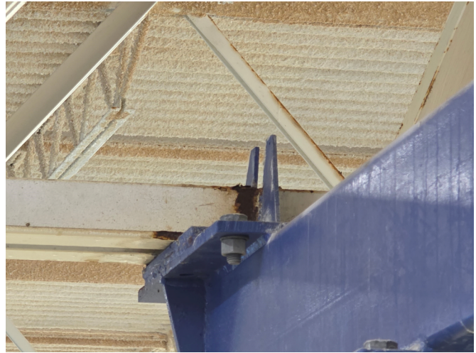
16. CORROSION ON ROOF/CEILING SYSTEM
