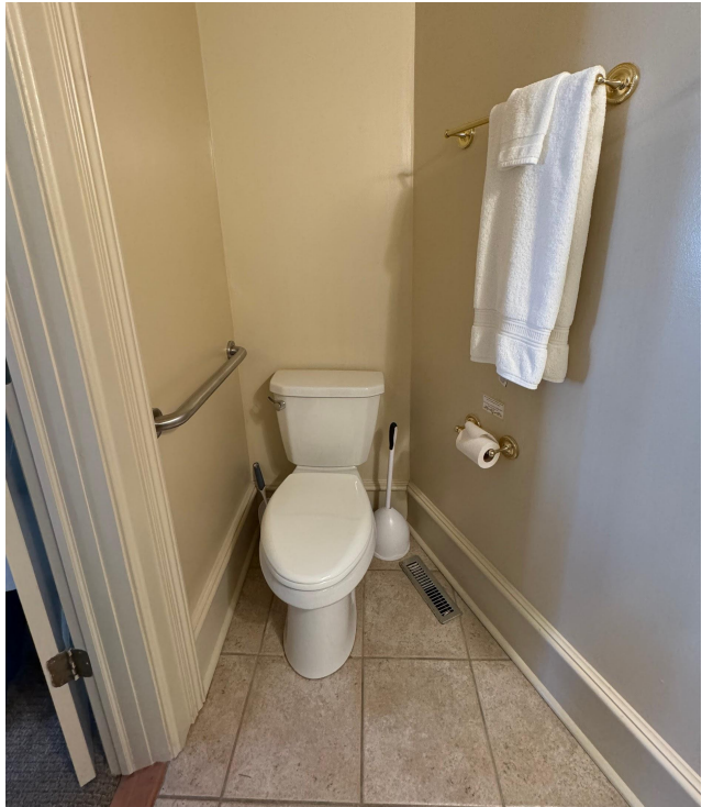
Need to add grab bars and remove towel rack
