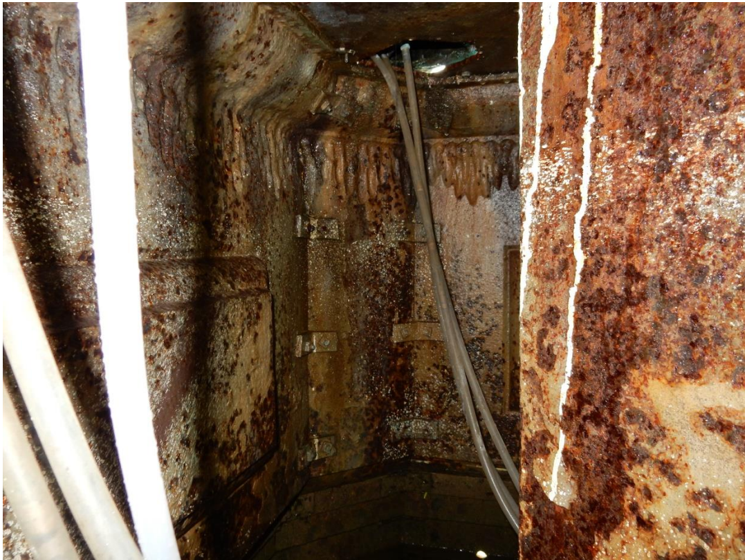
Image 06: Detail of Corrosion in Fountain Central Element
