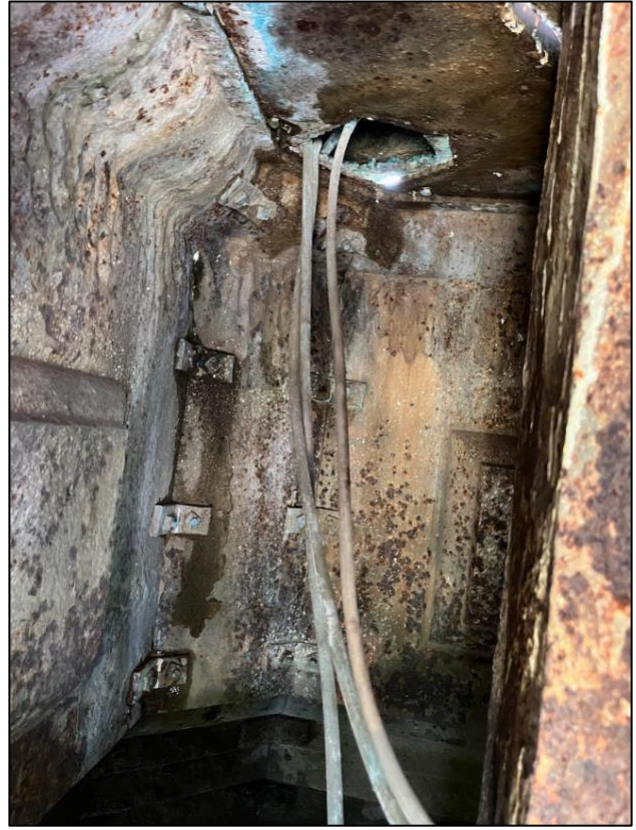
Fig. 2: Interior corrosion of the Birge Fountain
