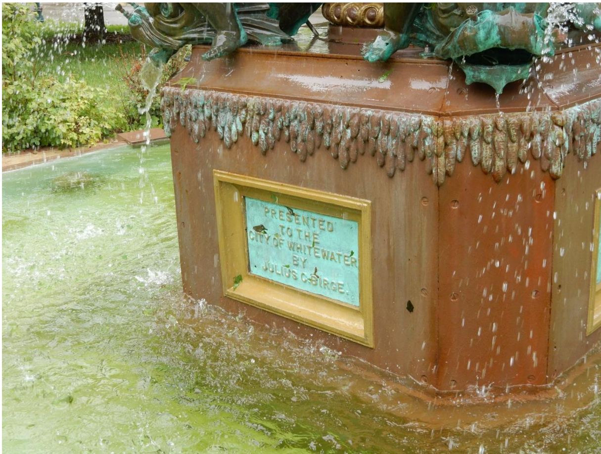
Image 04: Detail of Worn Coating
