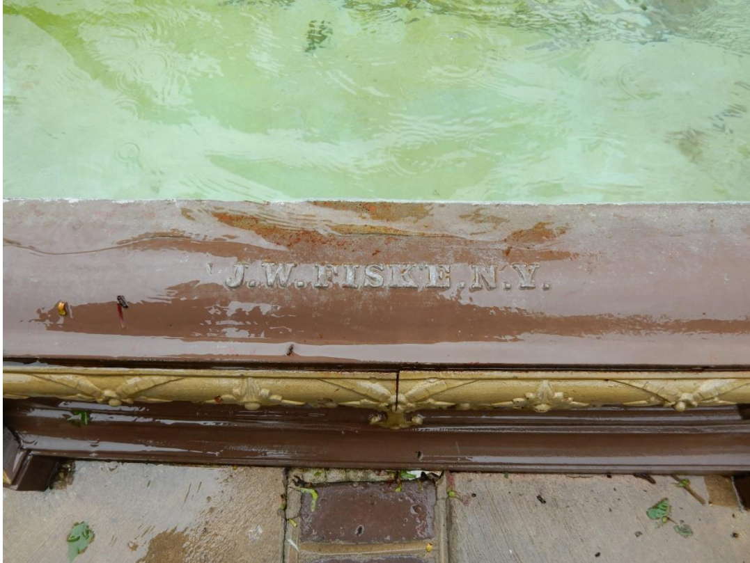
Image 05: Another Detail of Worn Coating; Manufacturer Name
