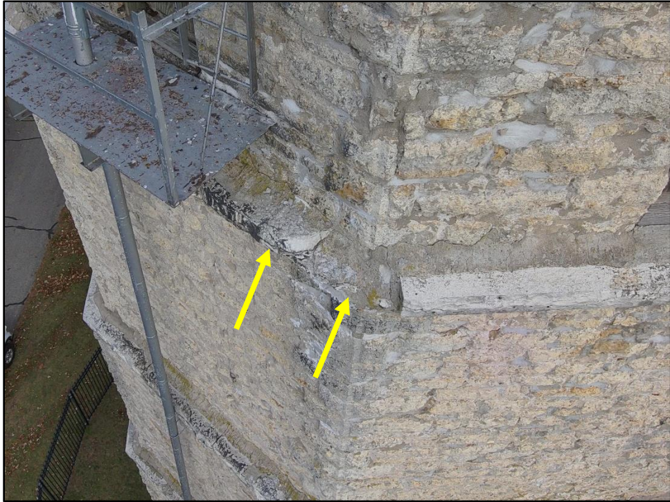
Photo 15: Missing stone, cracked stone, deteriorating mortar wash
