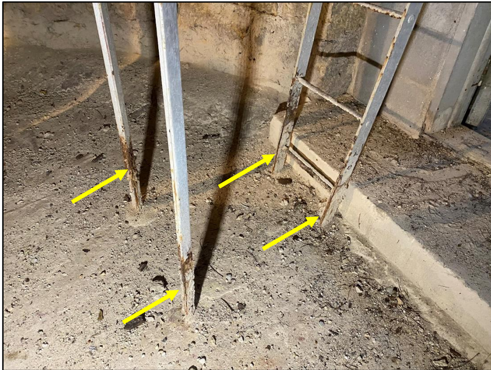
Photo 38: Base of interior ladder – corrosion on all pieces
