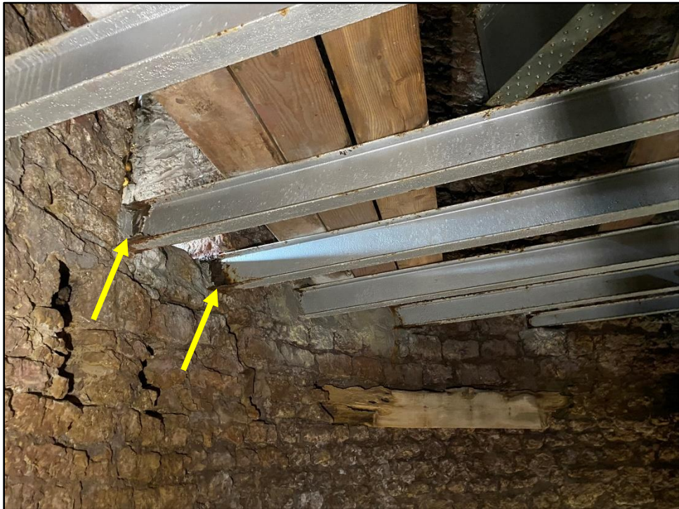
Photo 34: Signs of floor beam corrosion at walls
