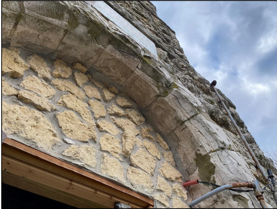
Photo 23: Cracked stone in entryway arch
