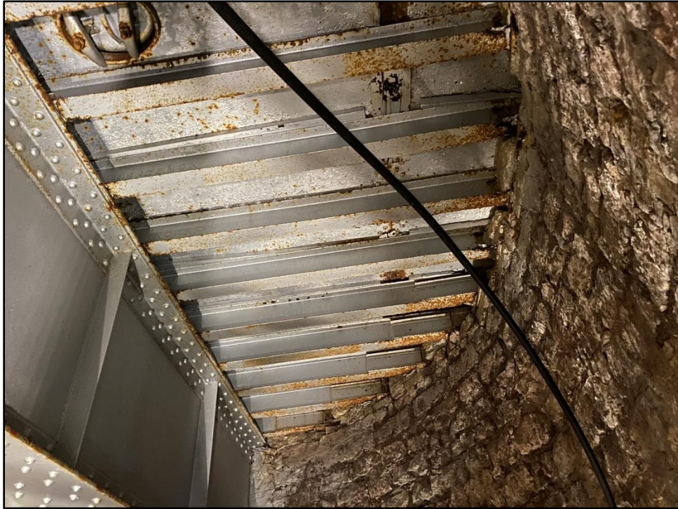
Photo 33: General surface corrosion of tank support beams with an increase near walls
