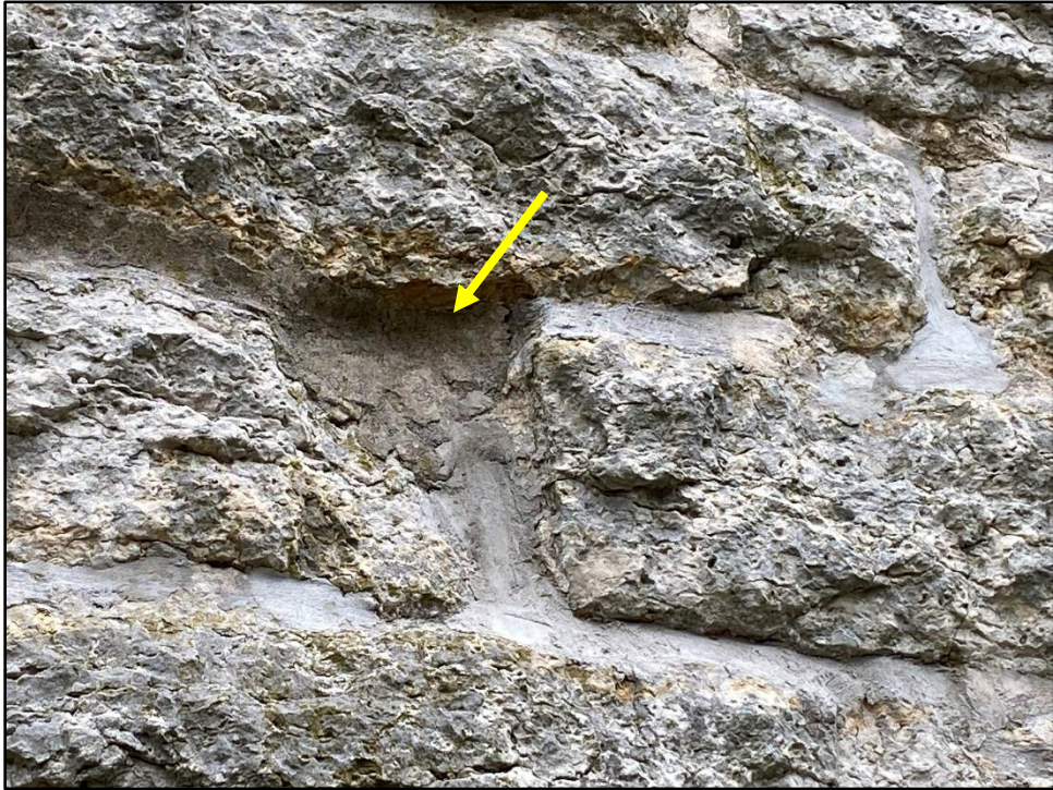
Photo 18: Isolated locations of stone spalls
