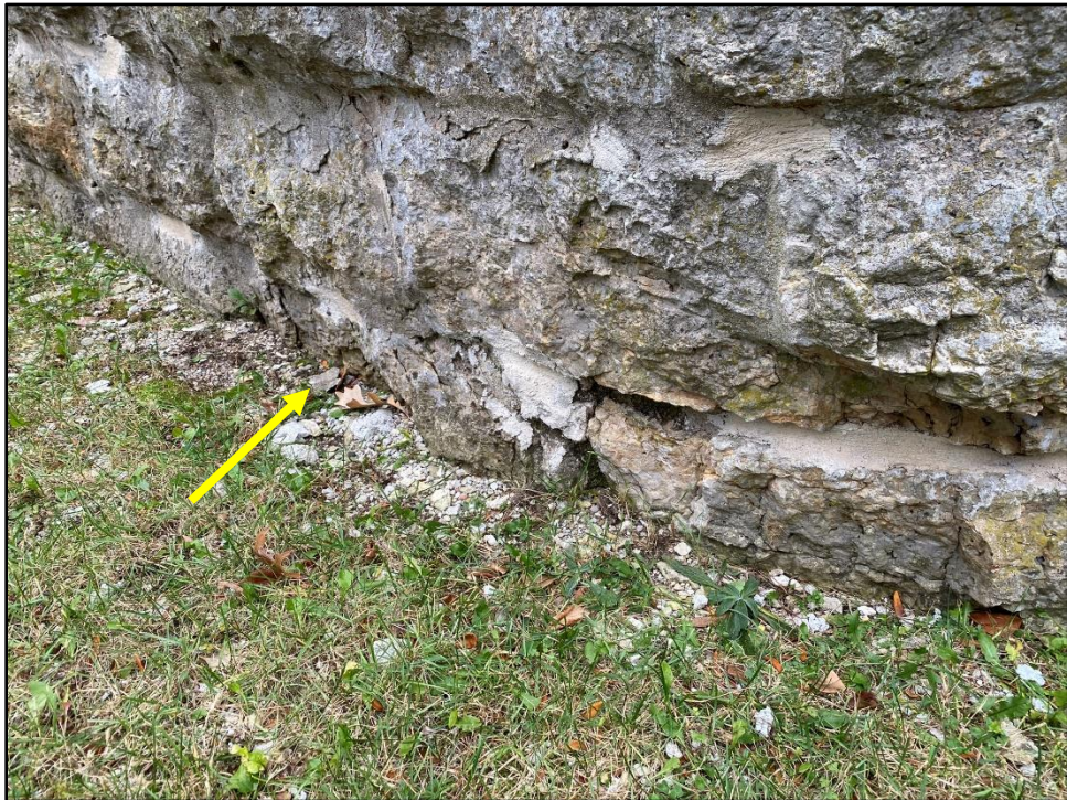
Photo 21: Stone deterioration at base of wall
