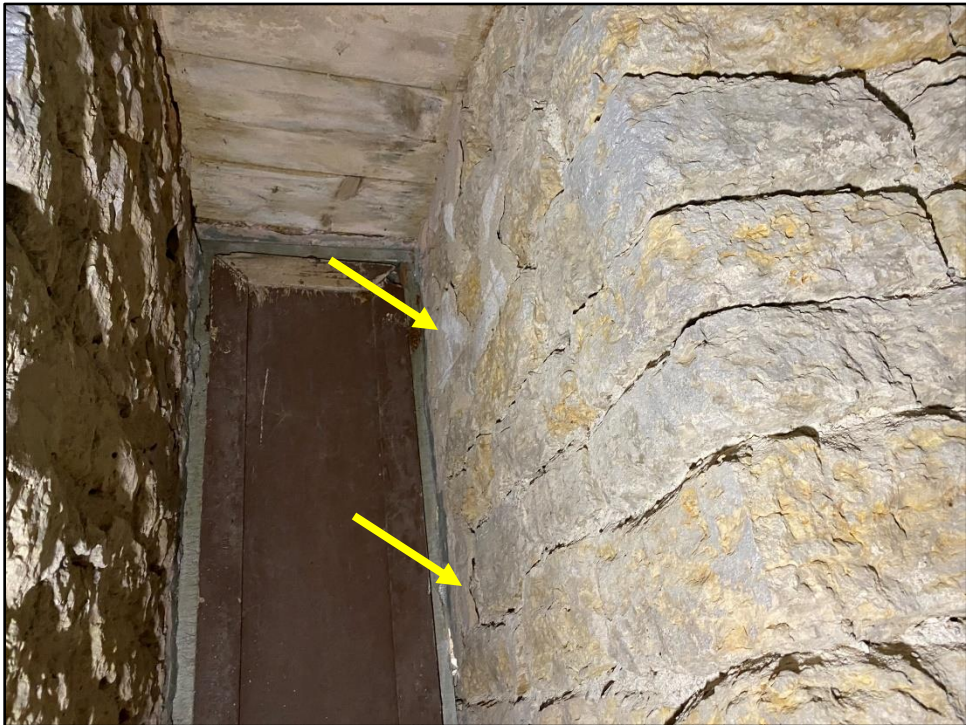
Photo 19: Spalled stone on "door" walls
