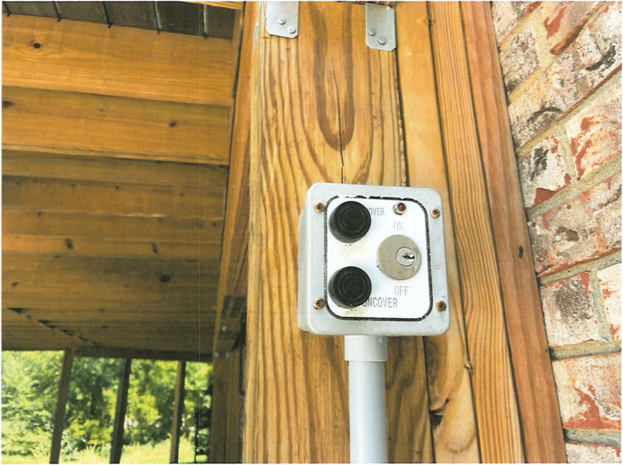
Figure D-2 – Keyed Control Switch (Key Removed)
