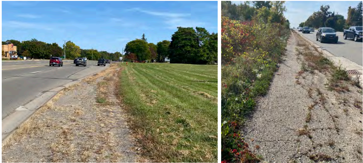
Aging and unkempt asphalt along edges of M-59
