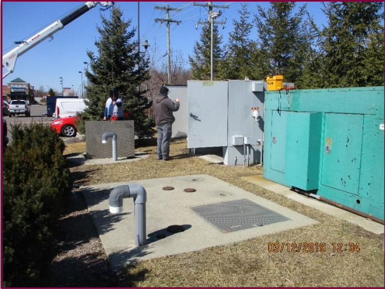
Village Lake Estates Pumping Station
