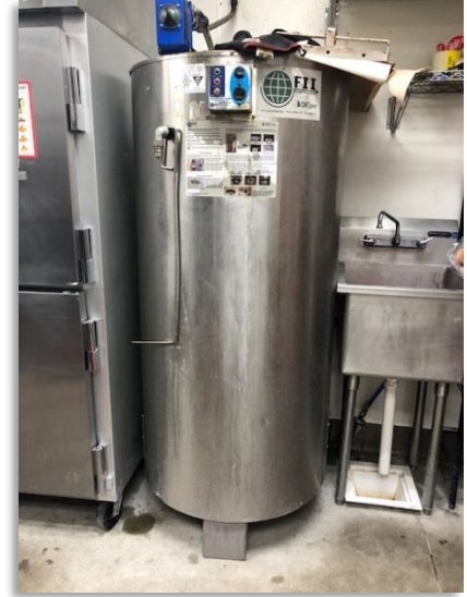
Grease Control Device at Sonic Restaurant
