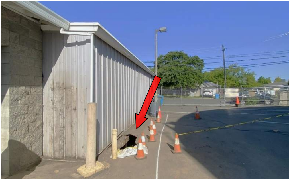
Photo 2: Location of Hole in Pavement (facing northwest towards 4 th Street)
