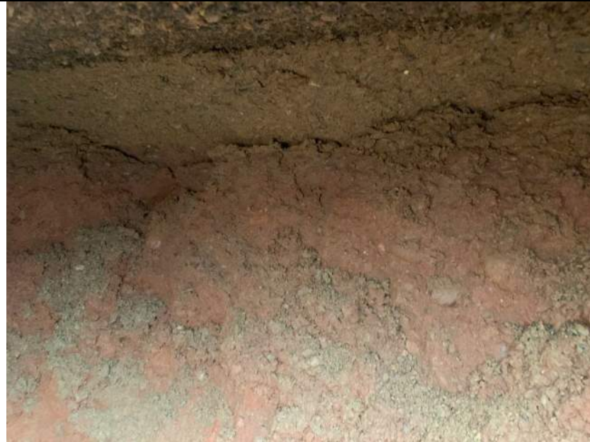
Undermined asphalt pavement at east edge of void. Bottom of AC is observed at top of photo.
