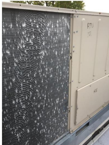
Damaged condenser coil fins.
