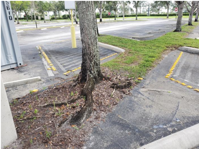
Example of 7" DBH Mahogany in narrow median with surface root damage to asphalt.
