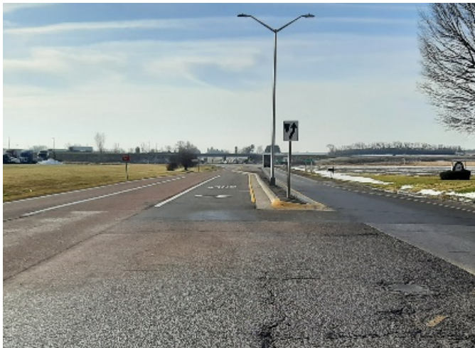
After Construction – New Left Turn Lane at S.T.H. 26 and Shaler Dr. intersection (Looking South)
