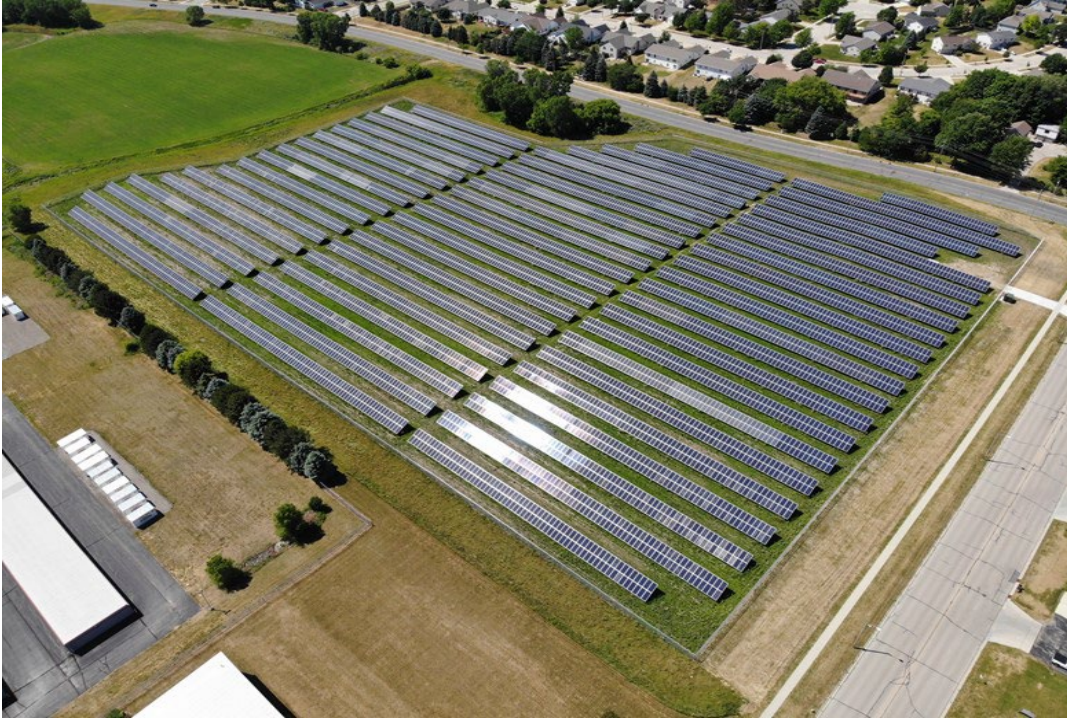
Figure 2 - Example of a solar array
