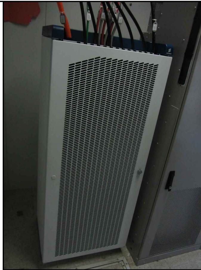
EXISTING LTE EQUIPMENT CABINET
