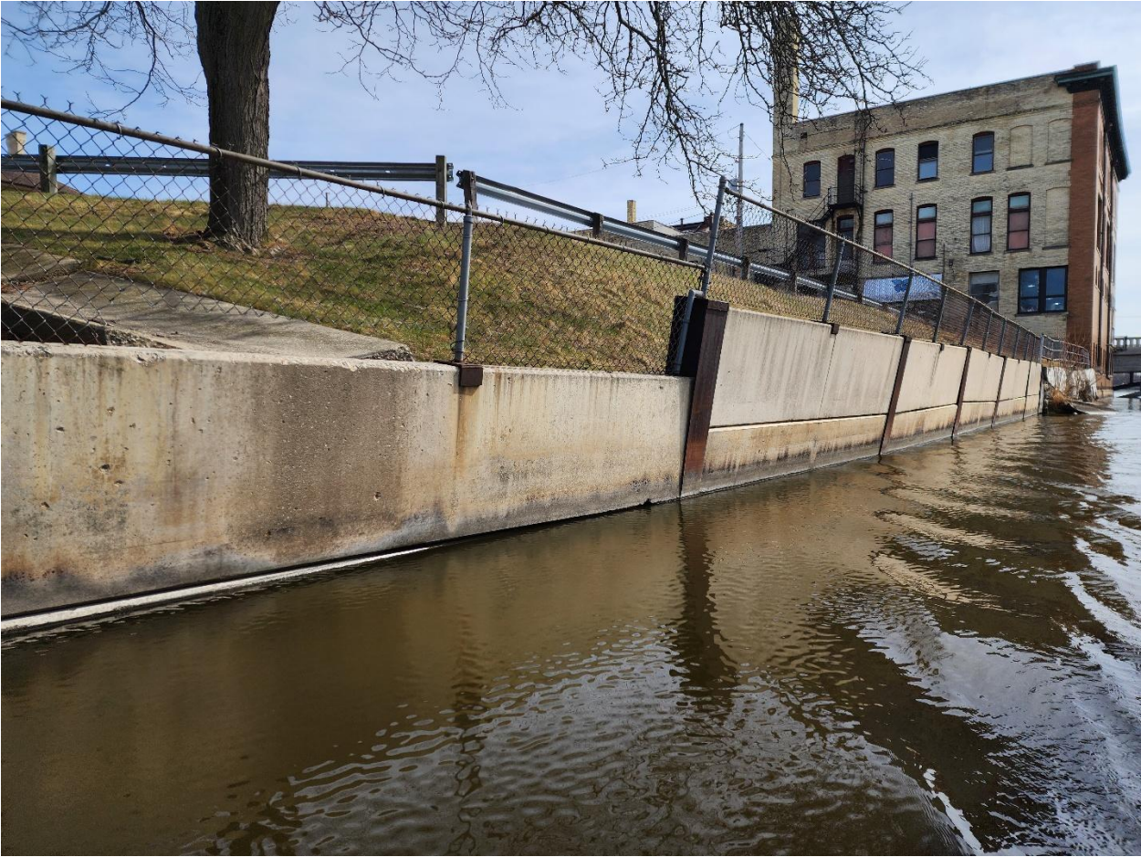
Figure 4. View of extreme deflection in Section B.
