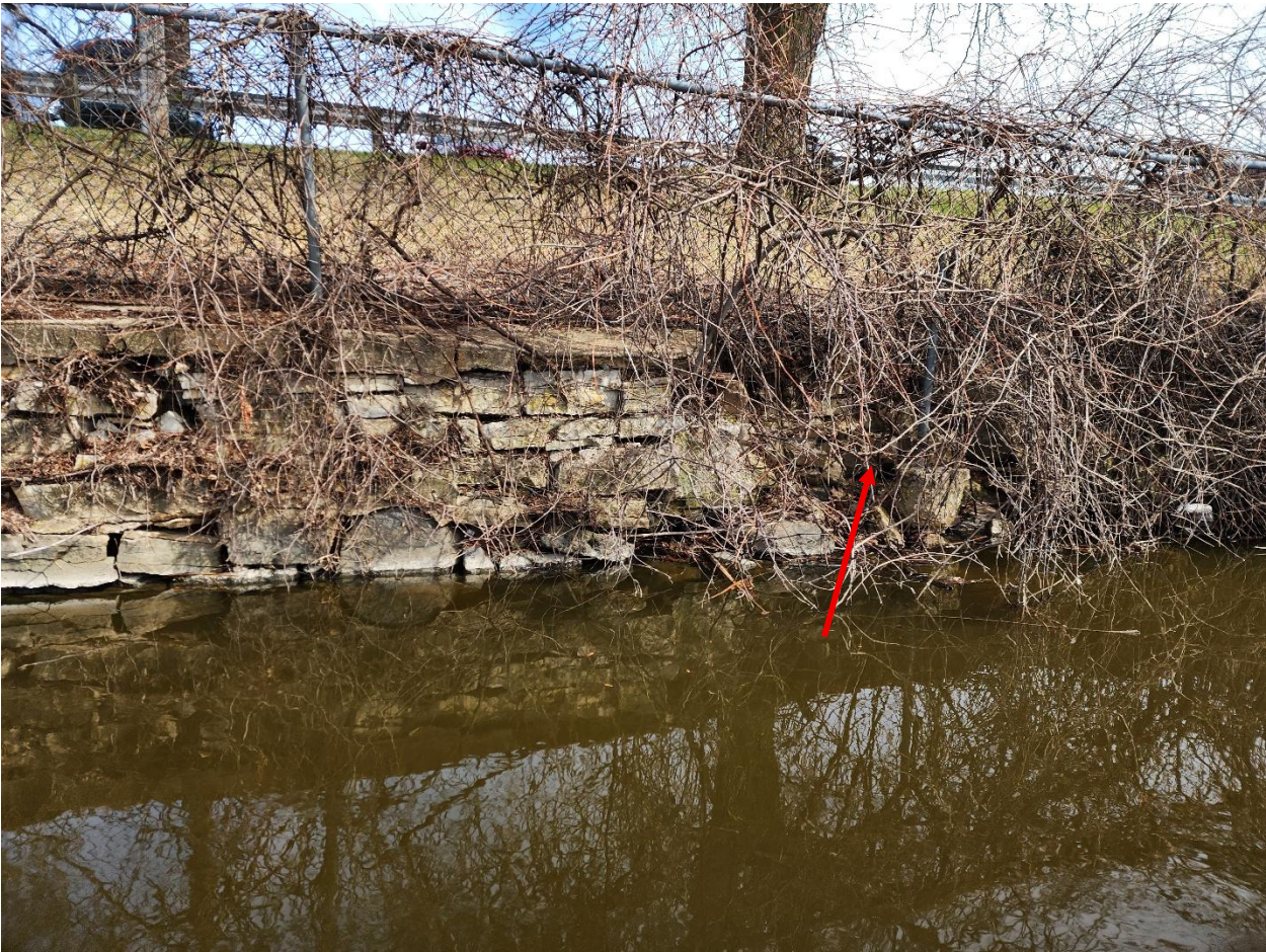
Figure 6. Failed portion of Section D.
