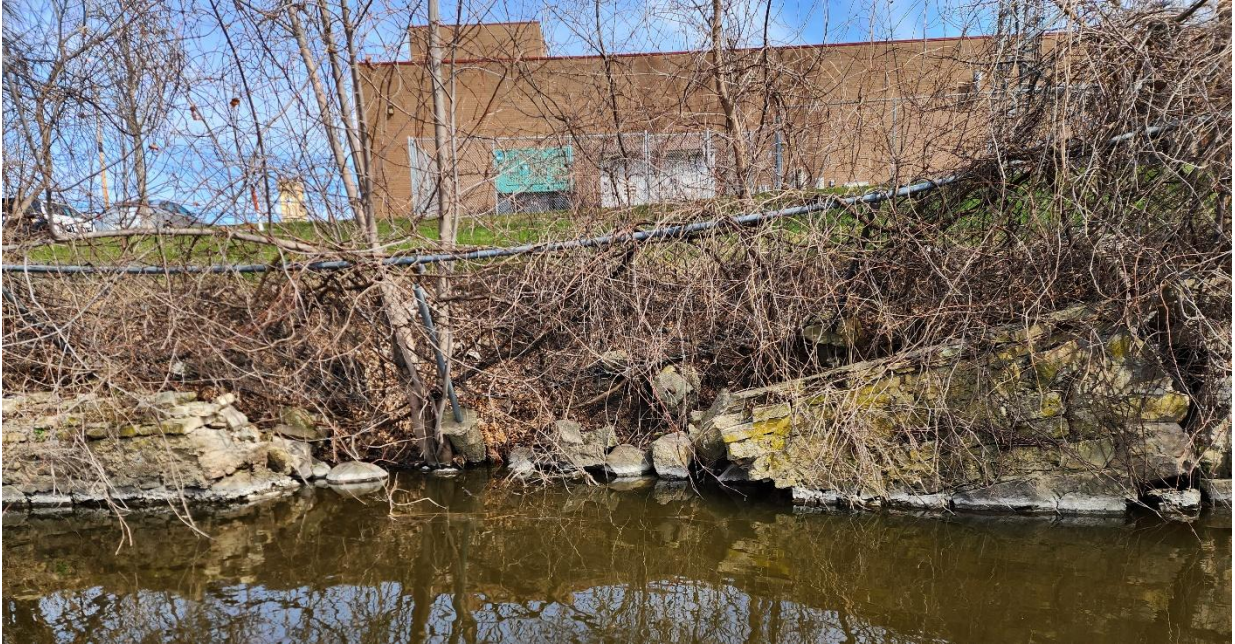
Figure 7. Failed segment of wall along Section E.
