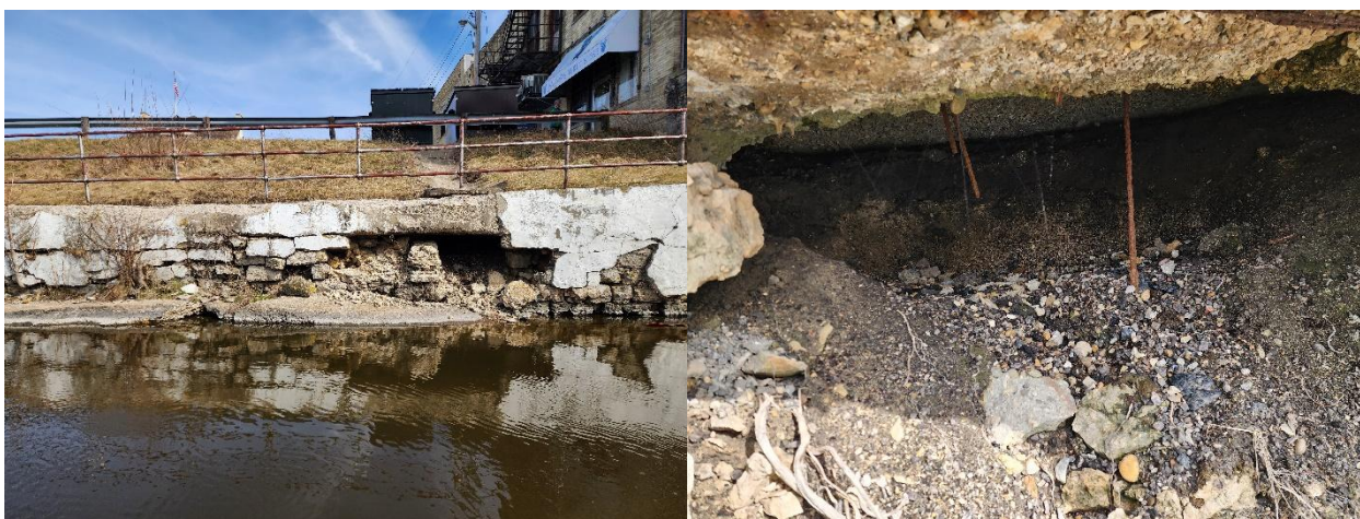
Figure 3. Location of void below surface drain (left) and depth of void (right).
