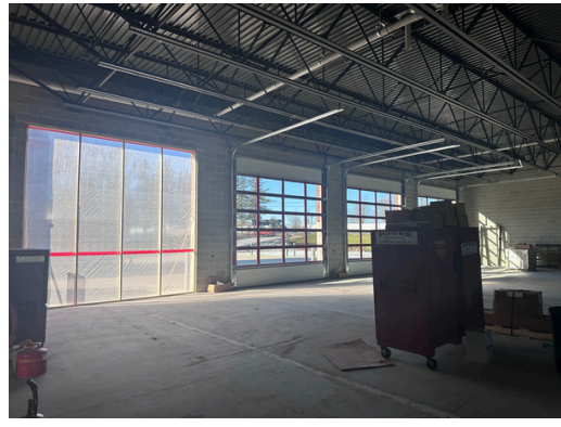
The apparatus bay doors went in. The first floor framing is mostly done.
