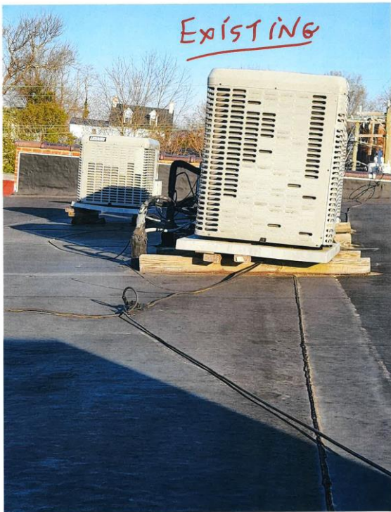
Existing Central System:
