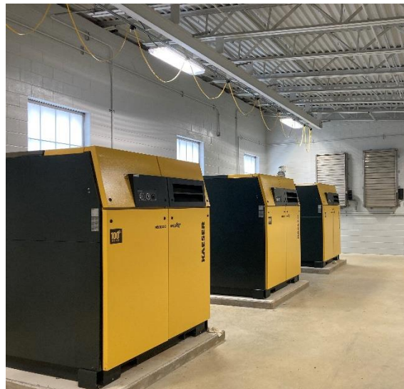
MBBR Aeration Blowers
