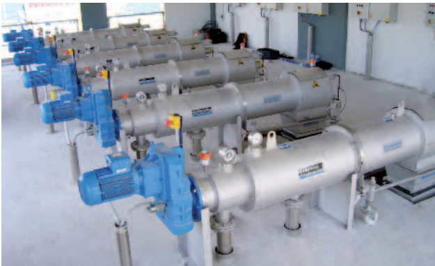
Sludge screening on WWTP Athens, Greece
