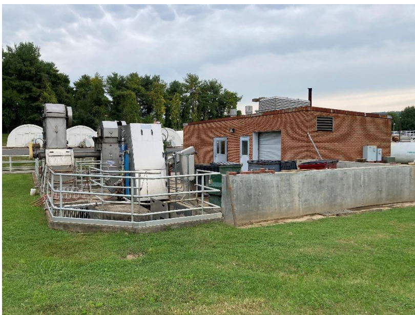
Influent Screen (foreground) and Grit Collectors (background)
