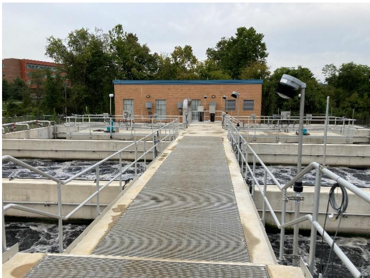
MBBR Process - Reactor Trains 1 and 2
