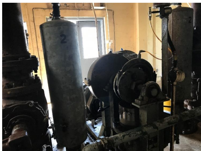
Sludge Pumps (primary and secondary sludge)
