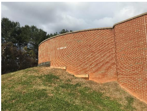
Primary Digester No. 1
