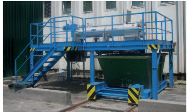
Outdoor installation of a HUBER Sludgecleaner STRAINPRESS®
