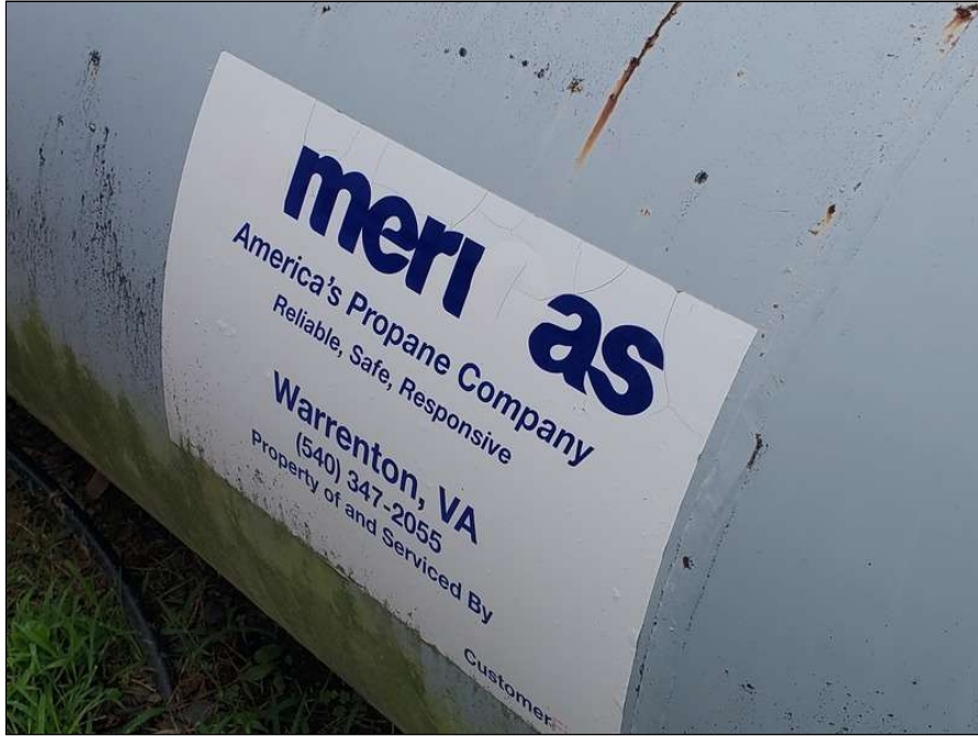
7 - Propane tank adjacent to utility building
