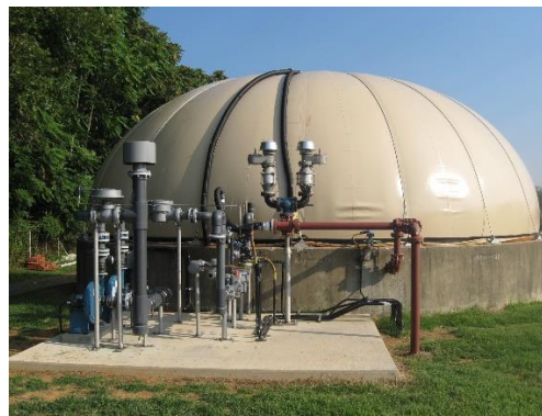
Digested Sludge Holding and Gas Storage
