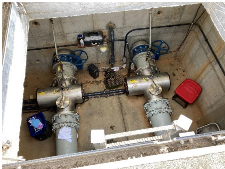
UV-disinfection In-line Reactors
