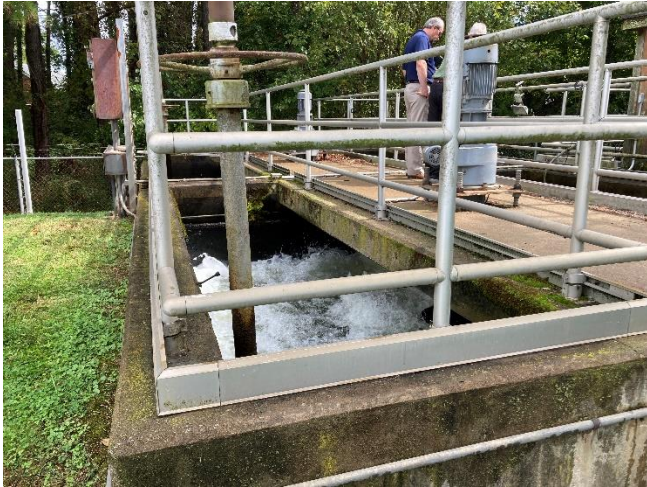
Post Aeration Tank and Surface Aerator
