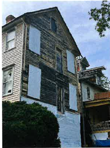
(Picture 11: Shows multiple doors with no fall protection, windows not maintained in good condition, wood rot and inadequate Roof drainage)
