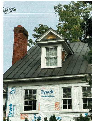
(Picture 6: Shows inadequate roof drainage, and inadequate protection from the elements)
