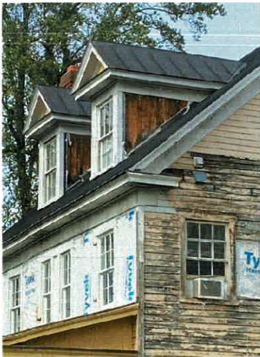
(Picture 4: Shows exposure to the Elements, wood rot, peeling Paint, and inadequate roof Drainage)
