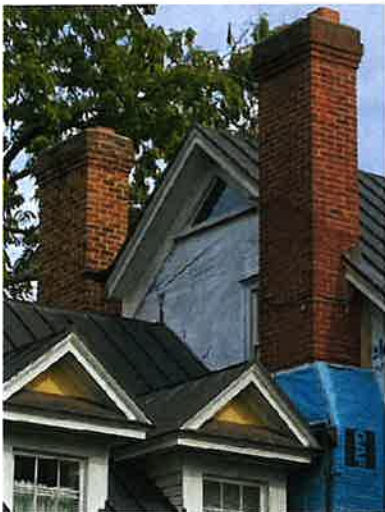
(Picture 7: Shows inadequate protection From the elements)
