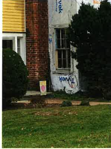
(Picture 13: Shows inadequate protection from elements)
