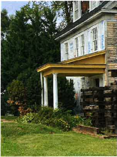
(Picture 1: Shows exposure to the Elements, rotted wood and inadequate roof drainage)
