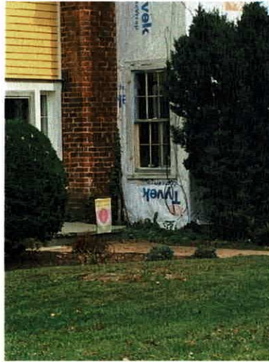
(Picture 13: Shows inadequate protection from elements)
