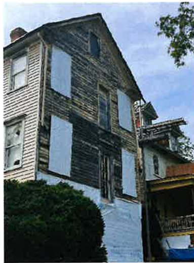
(Picture 11: Shows multiple doors with no fall protection, windows not maintained in good condition, wood rot and inadequate Roof drainage)
