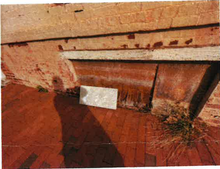
Picture 8: Shows missing window, exposure to the elements, rotten wood, peeling paint and damaged bricks.
