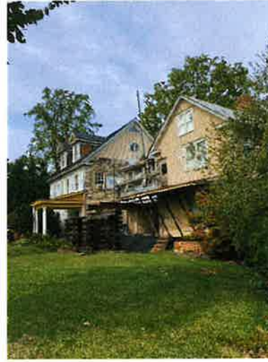
(Picture 3: Shows faulty structural supports, Inadequate roofing on right side, wood rot, and peeling paint)
