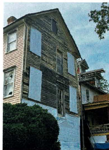
(Picture 11: Shows multiple doors with no fall protection, windows not maintained in good condition, wood rot and inadequate Roof drainage)
