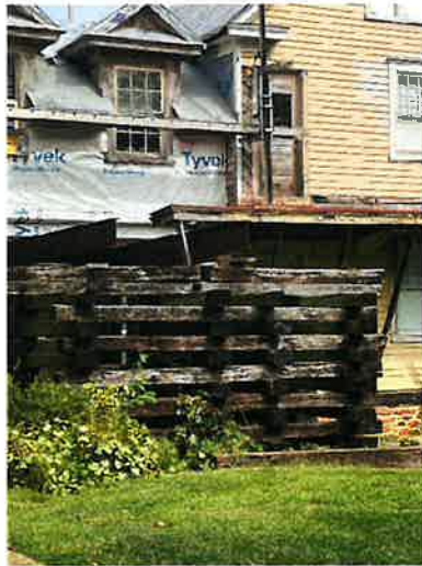
(Picture 5: Shows faulty structural supports, inadequate roofing, and exposure to the elements)
