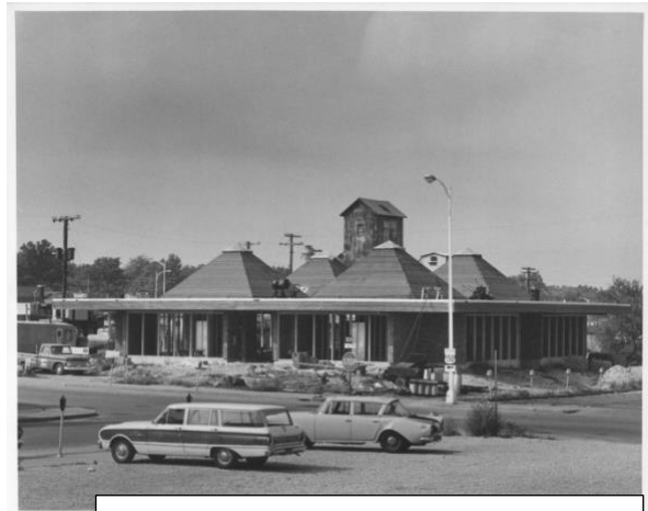
Under construction with the feed store behind. From the Champaign County Archives, vertical file
