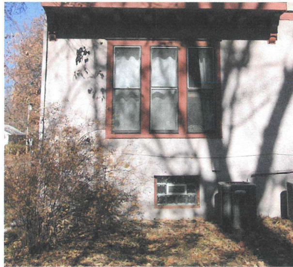
South elevation, first floor, west end. Smooth stucco water table, glass block basement window and 1/1 light sash windows.
