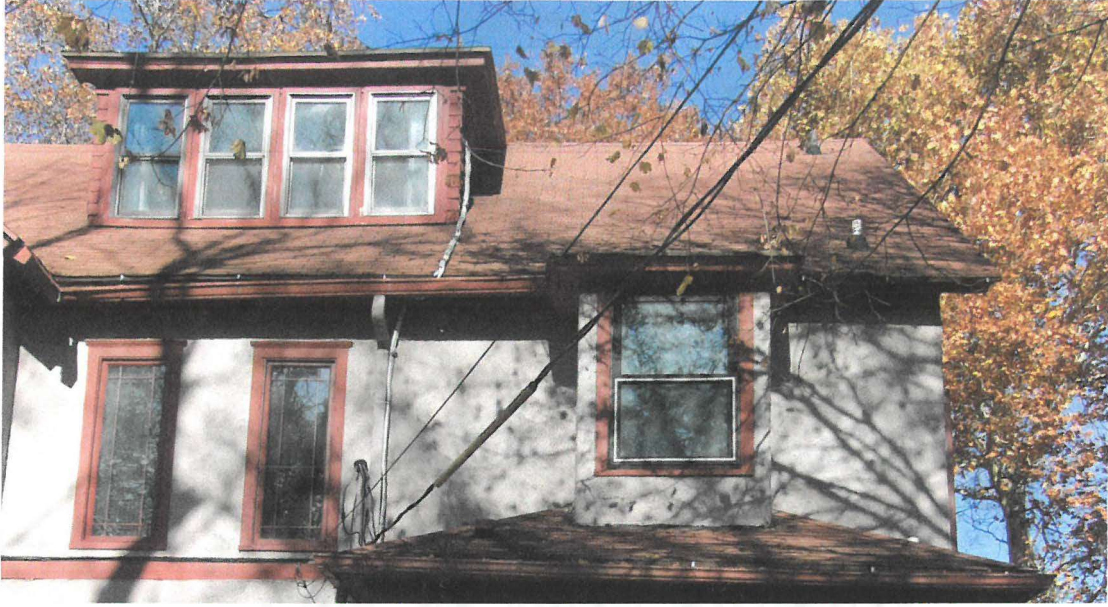
South elevation, second and upper floors, center and east end. Center, second story: two identical narrow single light fixed sash windows (above central staircase, interior). East end: narrow projection with low pitch shed roof atop first story pantry/kitchen entrance. A 1/1 light sash window occupies the center of this projection. Top story: shed dormer with low pitch roof and string of four 1/1 light sash windows.
