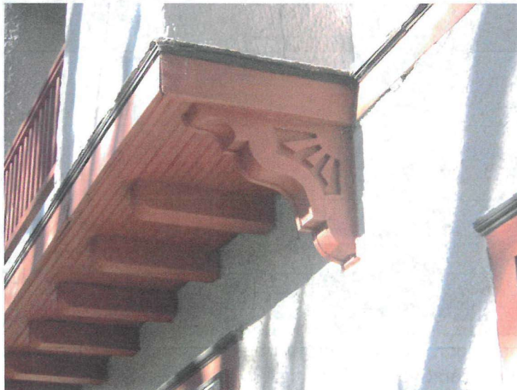
South elevation, second floor, west end. Projecting end gabled wall dormer, details.
