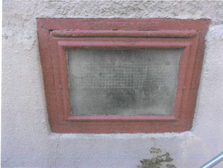
East elevation, center, water table. Majestic coal chute with wire glass door.
