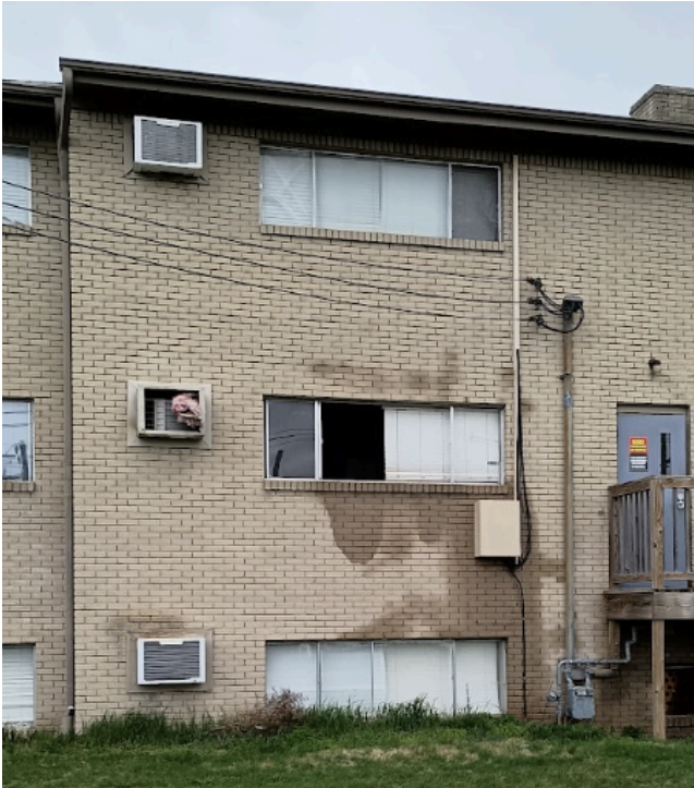
Water hazard near electrical
