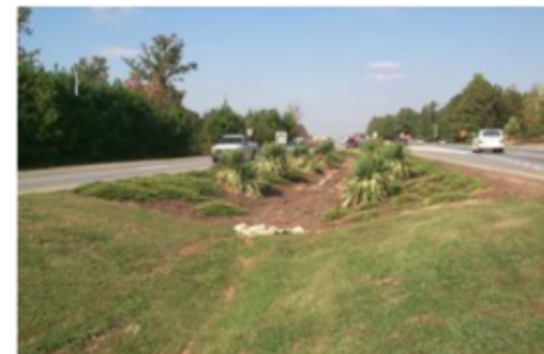
Enhanced Dry Swale
