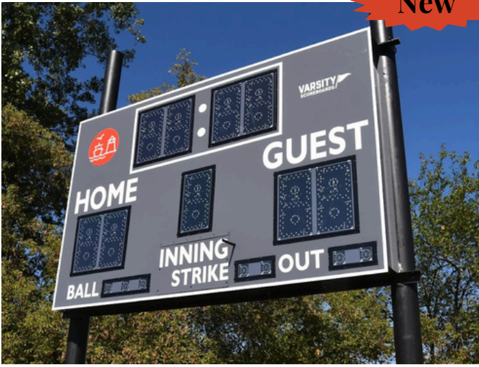
New scoreboards were installed on red and white fields which are primarily used for softball.
