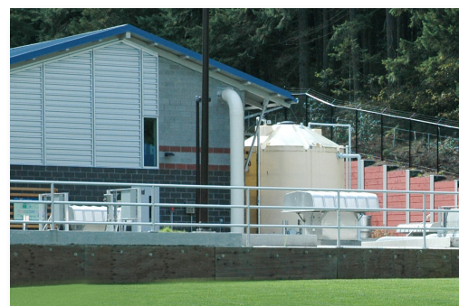
Martin Way Reclaimed Water Plant
