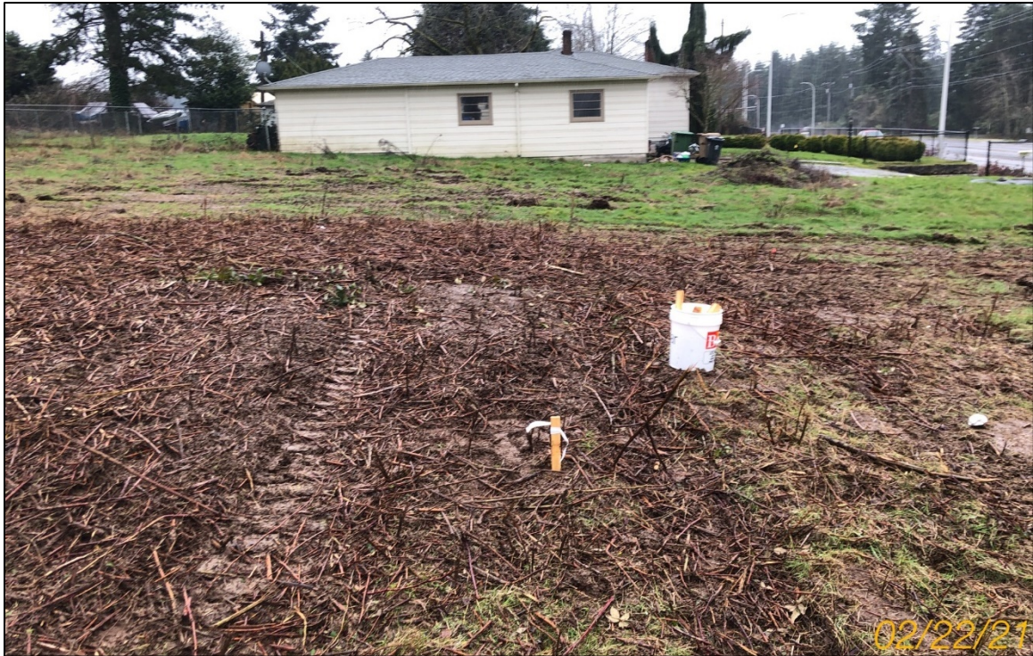
Photo 2: Looking south from the northwest corner of the project site at an existing house to be demolished.
